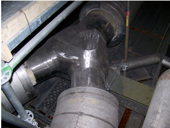
Fig. 6. A major heavy wall component tends to force all the thermal stresses into the pipe. Analysis tends to undercalculate the stress in the flexible pipe. Use extra conservatism.
