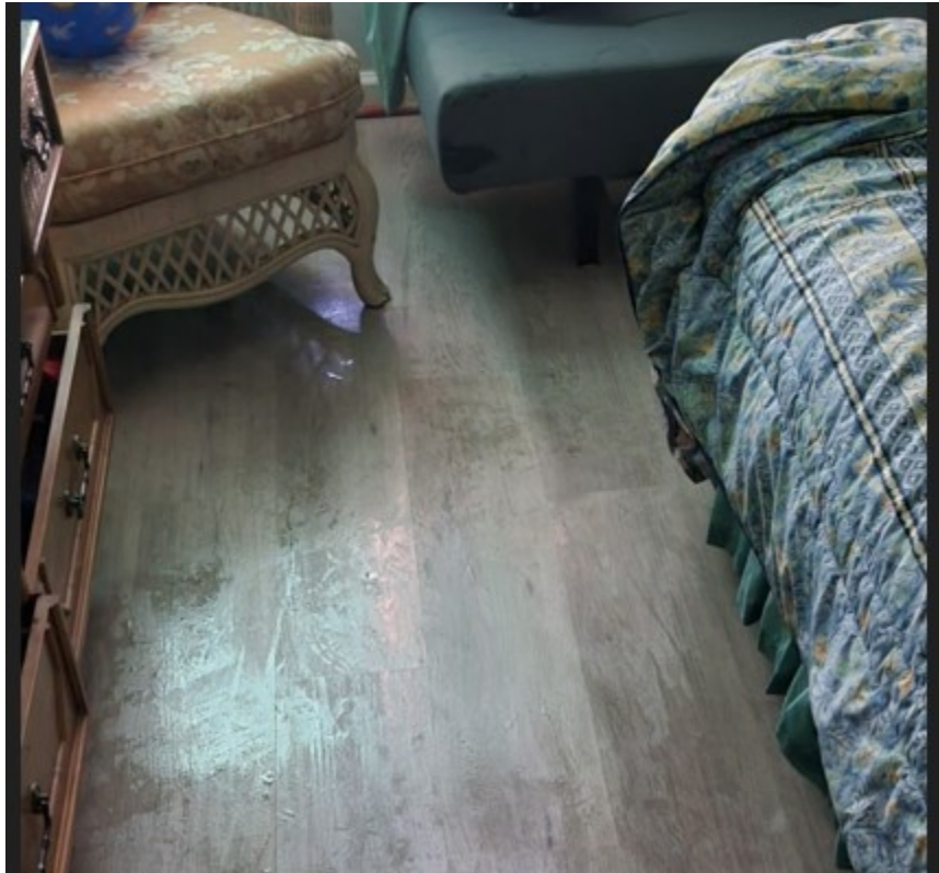
Flood water, which entered a residential dwelling.
