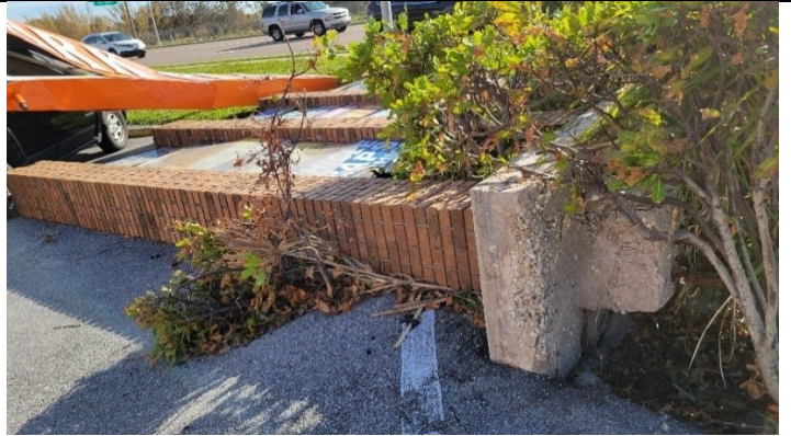
Shopping Center Sign failure
