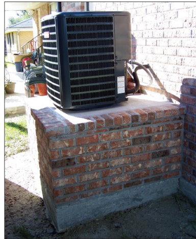
Figure 3-1. Air conditioning compressor elevated on a pedestal.
