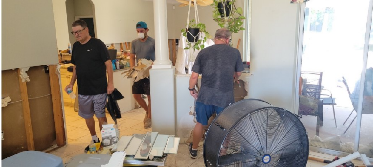
The bottom four feet of drywall are being removed by volunteer after the building was flooded.
