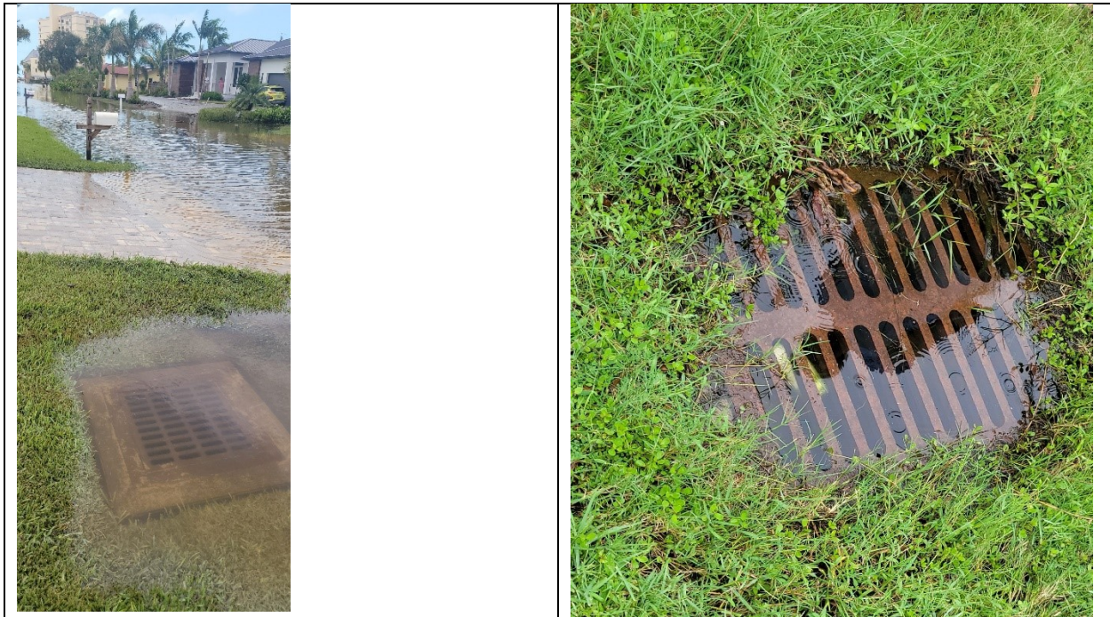
Inoperable catch basin due to clogging at the distant beach A field inlet backed up elsewhere
