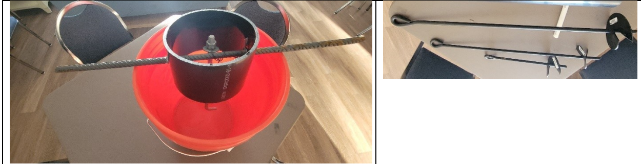
Rebar and anchor bolt form with bucket size pit to be dug
