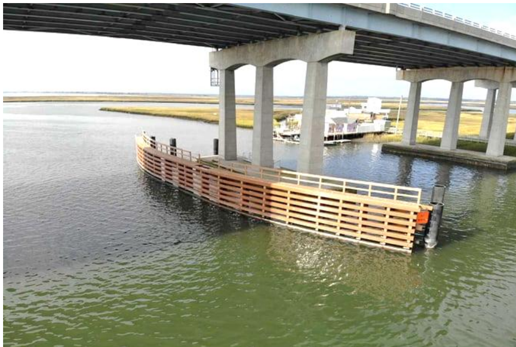
Figure 5: Fiberglass fenders to protect a bridge pier along a boating channel.
