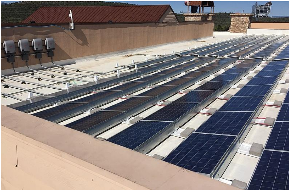
Figure 18: A ballasted photovoltaic panel system which is held down with blocks.
