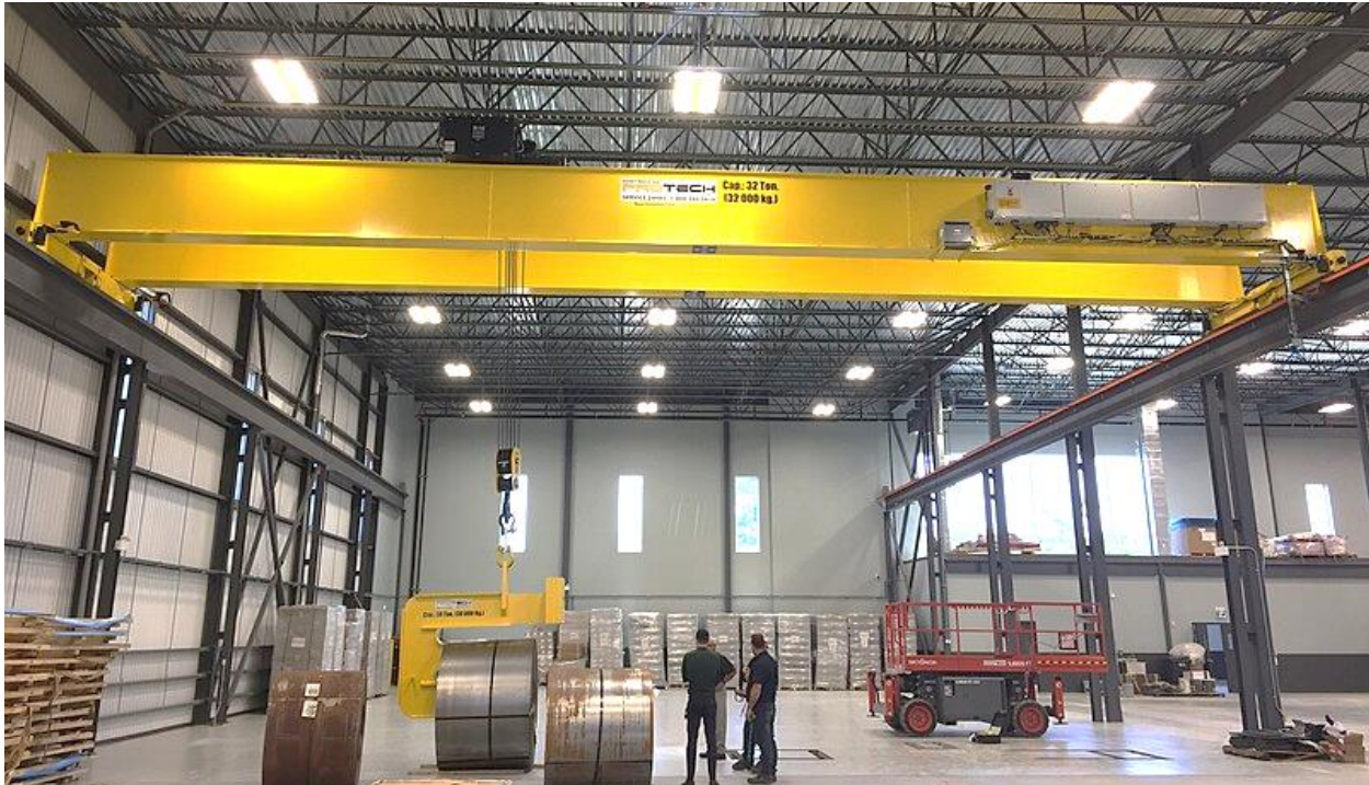
Figure 13: Overhead bridge crane that moves along rail beams.
