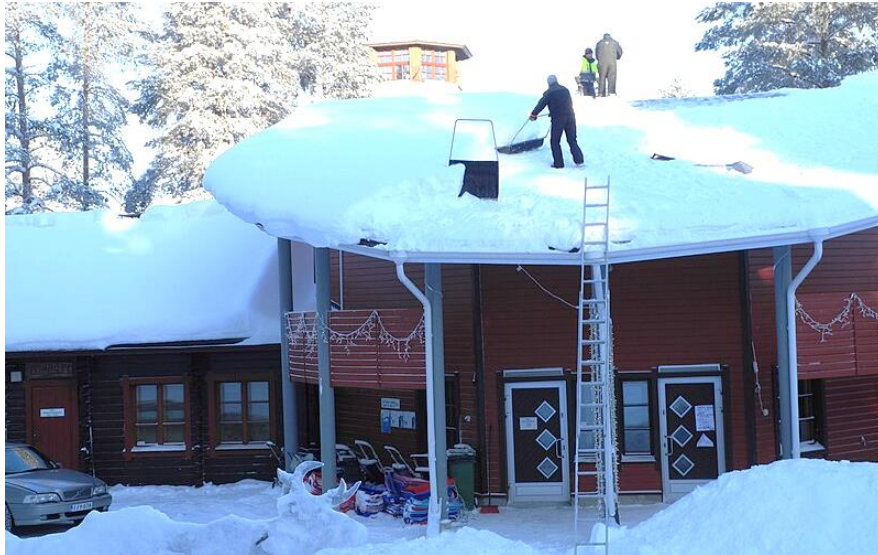
Figure 2: Snow buildup and snow drifts on a roof.
