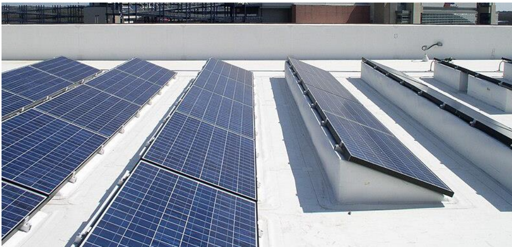
Figure 12: PV panel system (solar panels) on a flat roof with a tilt towards the south.
