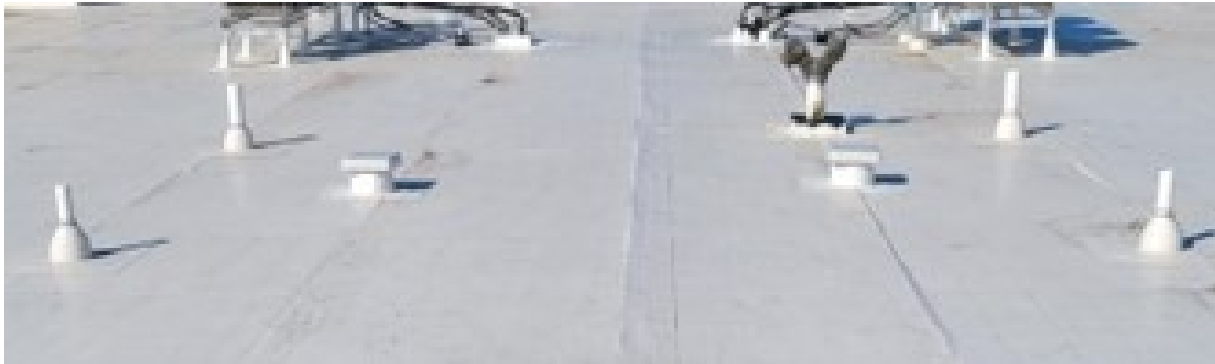
Typical TPO (thermoplastic polyolefin) single ply membrane with plumbing vents.
