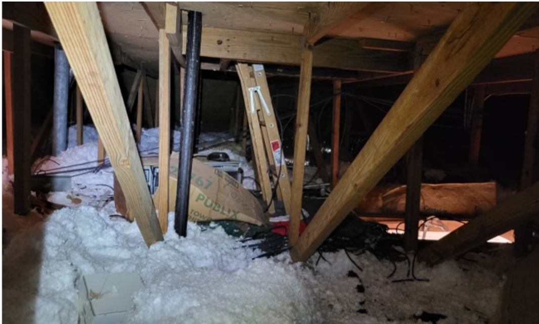
Roof trusses in attic crawl space with access hatch and blown in ceiling insulation.
