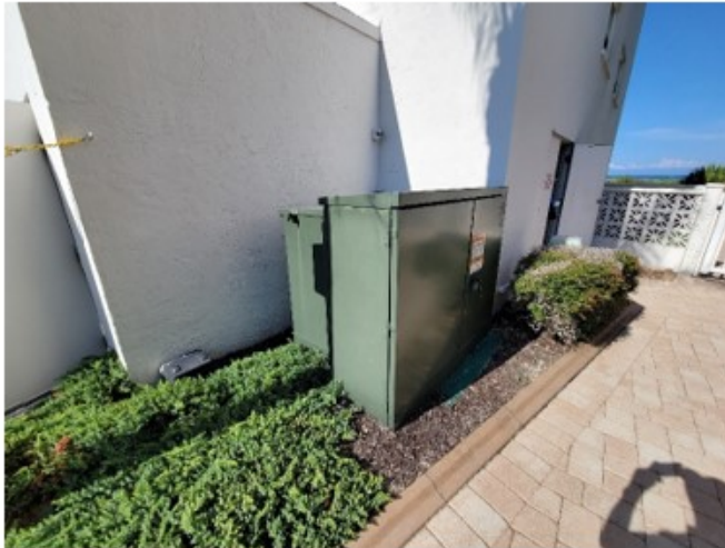
Electric transformer box – responsibility of Florida Light and Power not condo.
