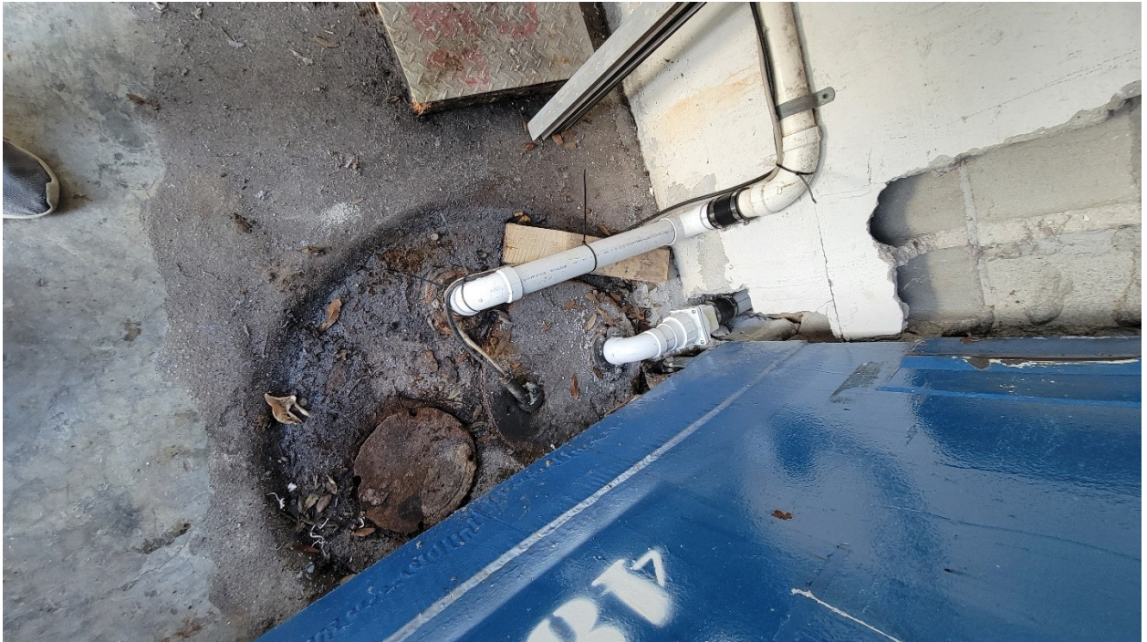
Trash room sump pump would be the Association's responsibility.
