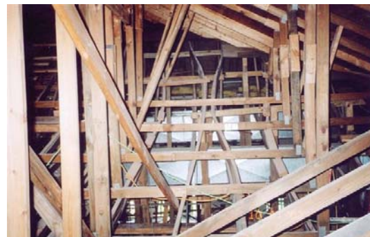
Figure 3: Buckled truss top chord
