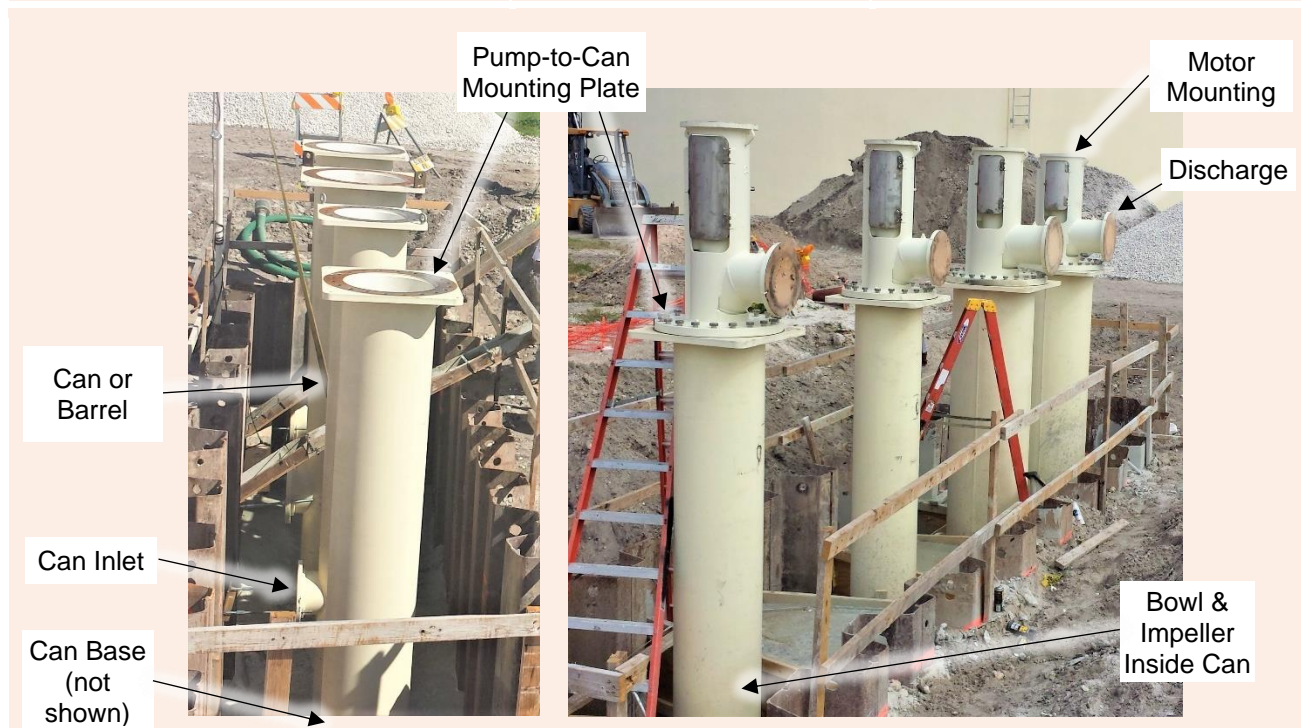
Figure 8: Four vertical can pumps (a.k.a. barrel pumps) prior to encasement in concrete. Left: Cans installed without VS1 pumps. Inlet manifold piping also needs to be installed. Right: After VS1 pumps set into the cans and bolted to the mounting plates.
