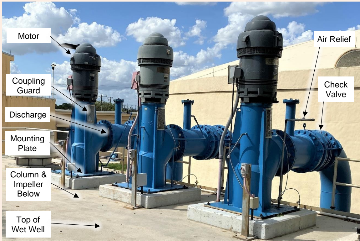
Figure 5: Three axial flow pumps mounted on top of a wet well for transferring water to a storage tank. An axial flow pump is similar to a mixed flow pump, as shown in Figure 4, except it has an axial flow impeller as shown in Table 1.
