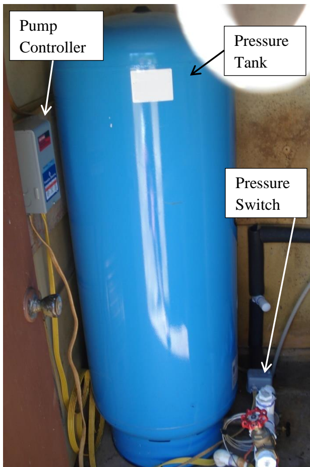
Left: An 81 gallon Flexcon Industries Flex2Pro H2P80 pressure tank in a well house. Pressure tanks store water and keep the water under pressure so that well pumps don't have to kick on each time water is used.
