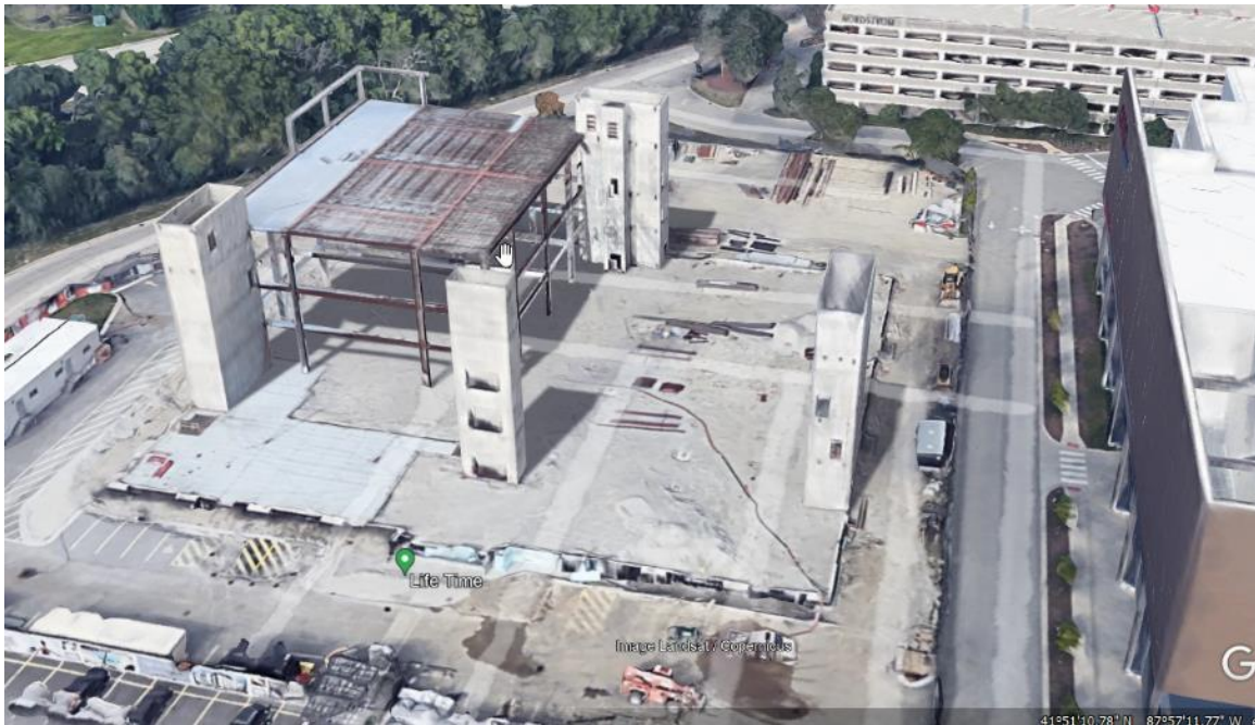
Fig. 9b, Athletic club under construction at a mall where there is insufficient room for the sequencing of tilt-up walls (Google Earth)
