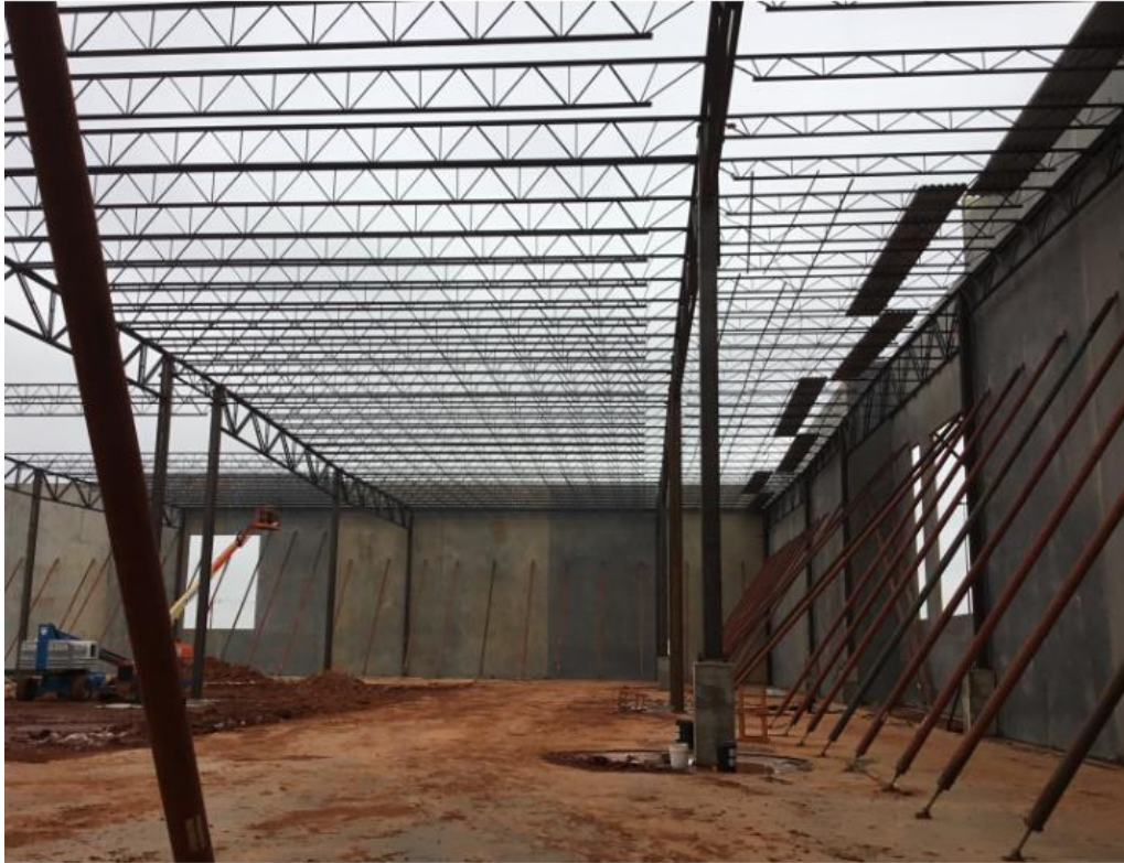
Fig. 46: Roof steel being erected with braced panels: Panels to remain braced until roof deck fully welded to steel joists and walls for diaphragm action.
