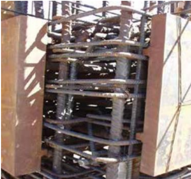
Figs. 27a, 27b Clearance between headed studs and rebar can be a real challenge at embed plates (Klinger, et al)
