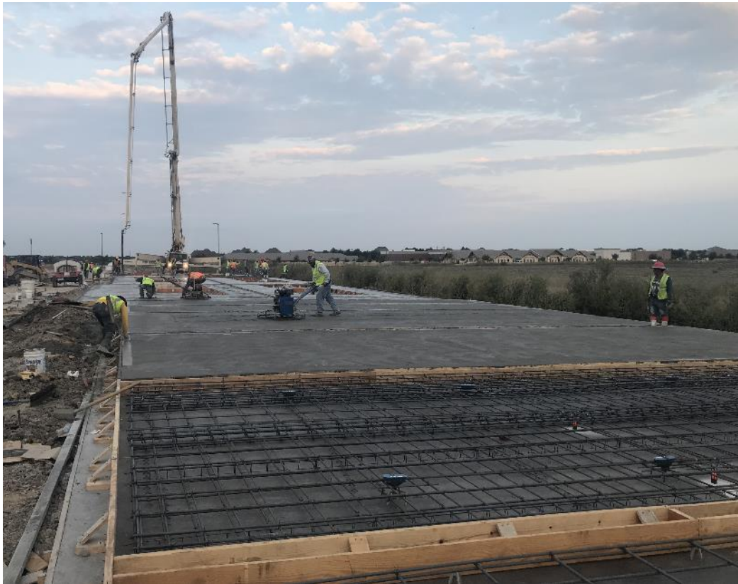
Fig. 4, Panels in various stages: Finishing of poured panels, and panel ready for pour
