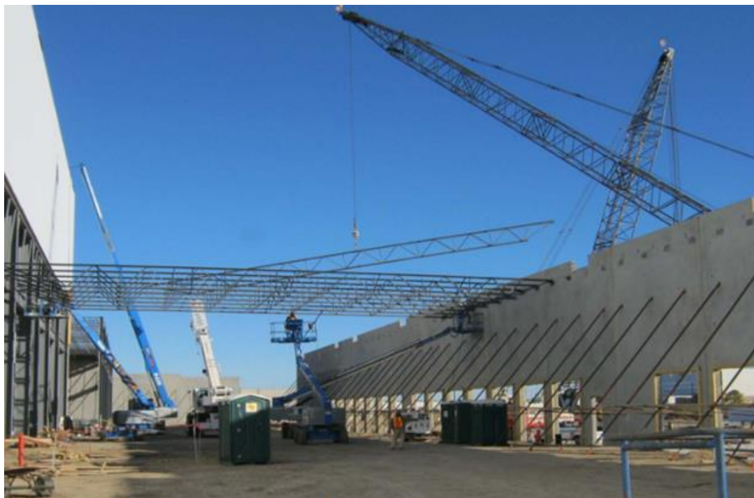
Fig.16: Inside view of loading dock area with steel roof joists bearing on tilt-up panels
