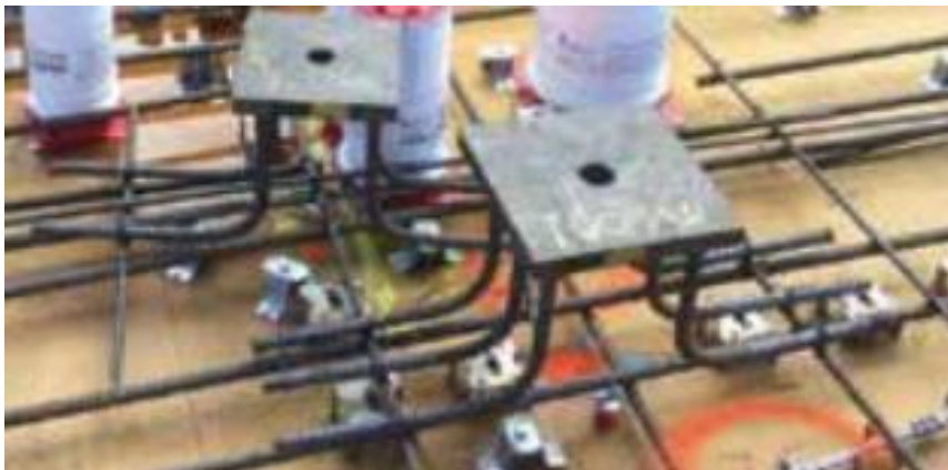
Figs. 26a, 26b, 26c: Embed plates for panel connection; Headed studs and A706 weldable rebar are options (Klinger, et al, and Author)
