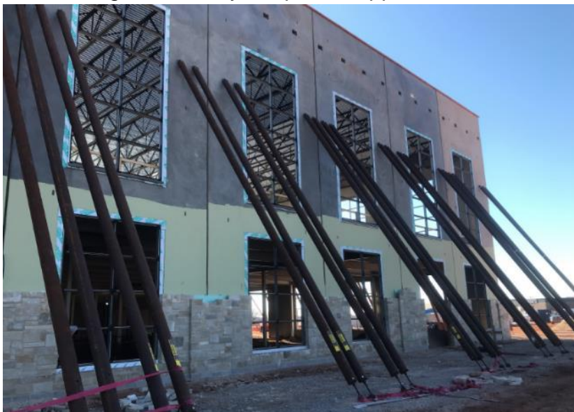
Fig. 43: Braces for two-story panels with a second story gym with large openings
