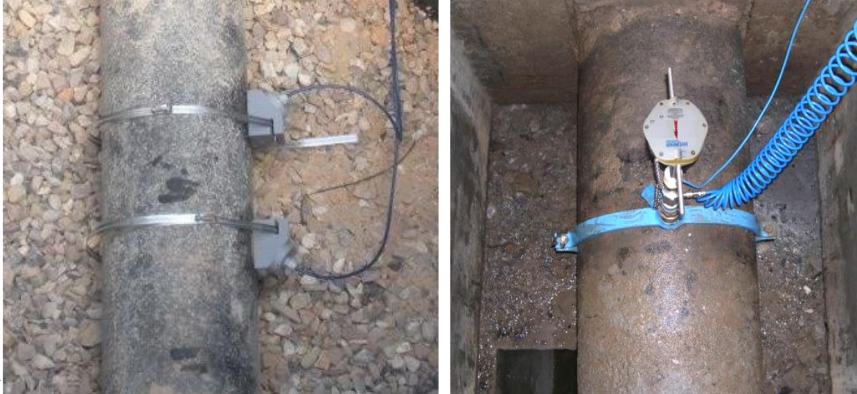
Figure 17: Examples of a strap-on ultrasonic flow meter (left) and a magnetic insertion meter (right), both installed on existing water mains.
