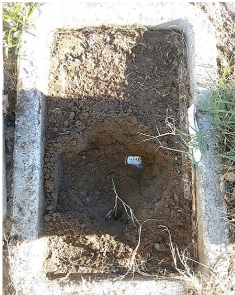
Figure 11: A buried manual water meter. The meter box should be Cleanout out to allow taking a meter reading.
