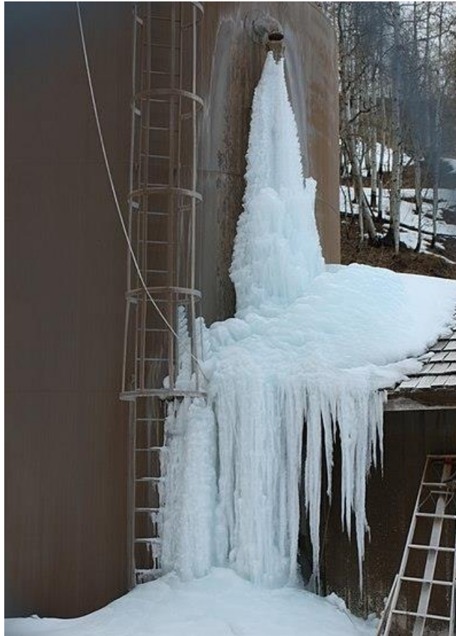
Figure 12: A ground storage tank with an overflow pipe and ice buildup leaving evidence of a recent overflow event.
