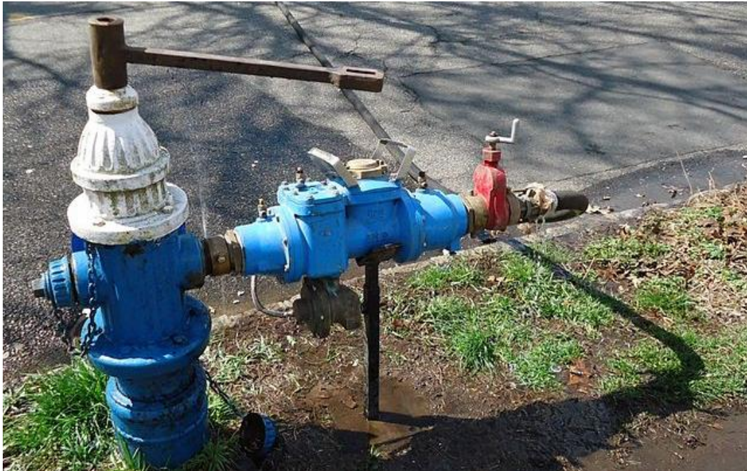
Figure 10: An authorized fire hydrant connection with a flow meter and backflow prevention device. This is an example of unbilled, metered, authorized consumption.
