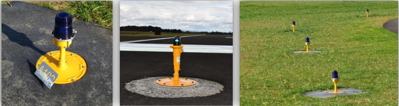
Runway & Taxiway Lights
