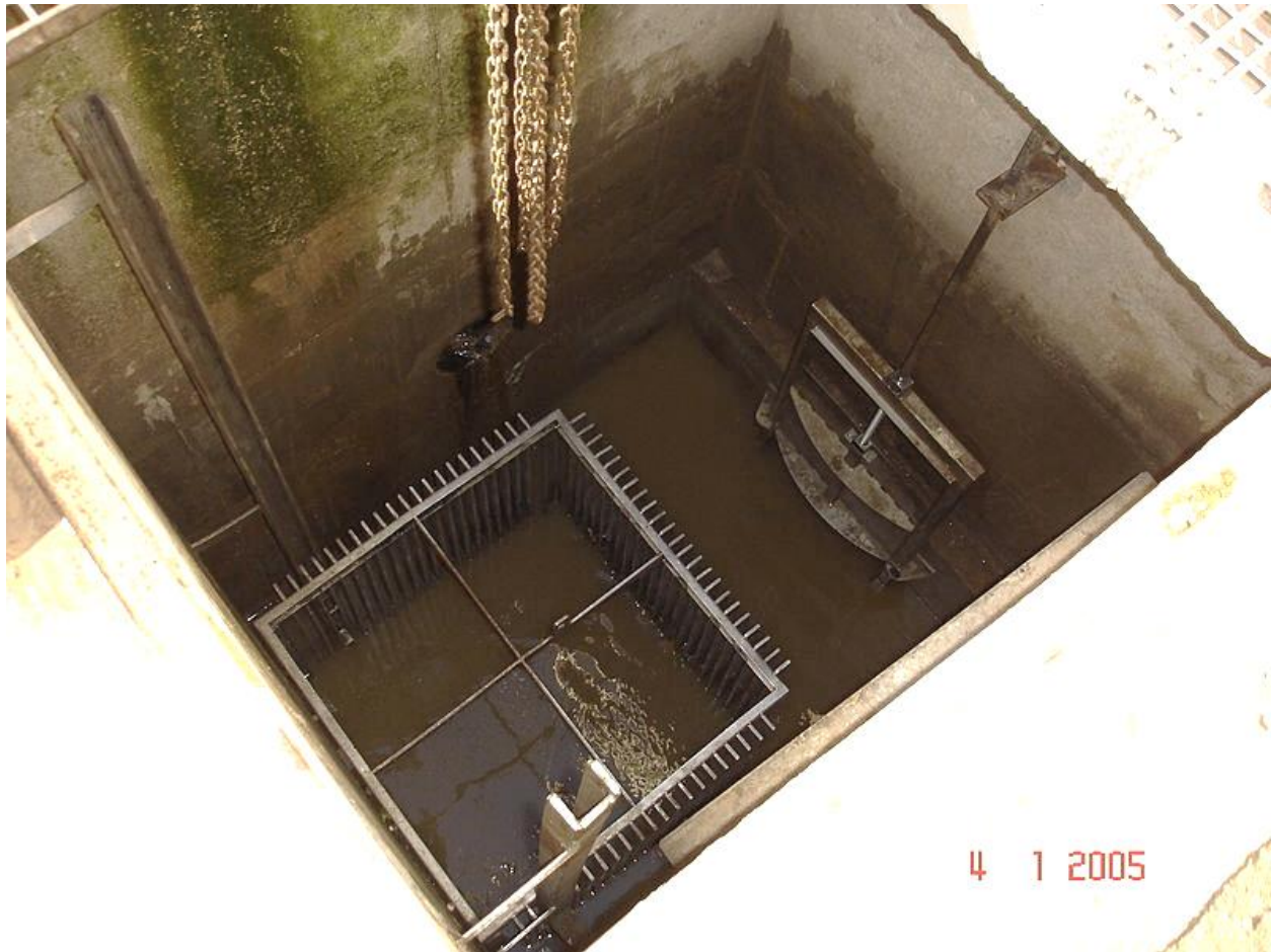
Figure 2: Example of a wet well with a basket screen, as part of a small industrial pretreatment system with primary treatment.
