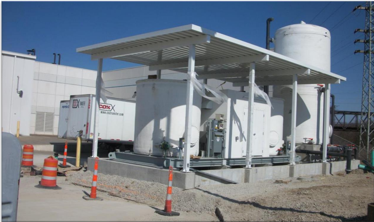
Figure 5: Example of a manufacturing facility with a pretreatment system circled in white (top) and at ground level (bottom). The system includes a large equalization tank and a pH neutralization system.
