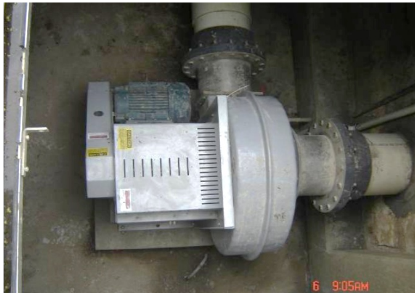
Figure 18: Looking down on a blower that draws odorous air from the right and discharges the air at a higher pressure through the pipe at the top.
