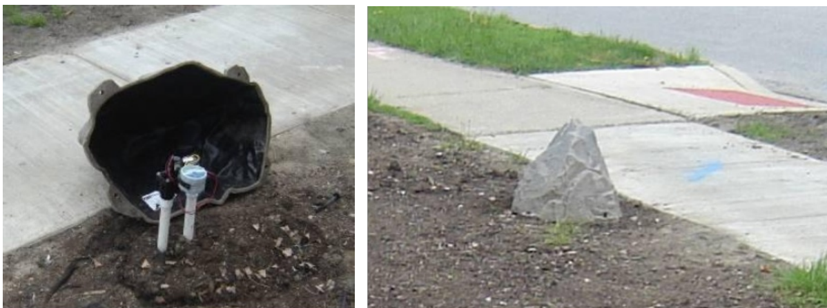
Figure 20: Irrigation valve and backflow preventer concealed by an artificial rock.
