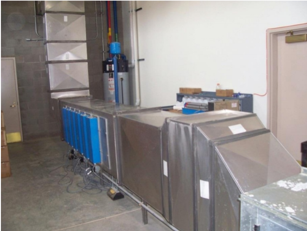
Figure 4: Example of an ionization odor control system. Inside the duct at the blue modules are a series of ion tubes.
