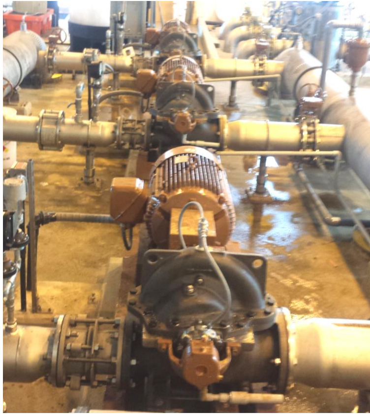
Figure 14: Three horizontal split-case pumps drawing from a suction manifold on the right and sending flow into a discharge manifold on the left.
