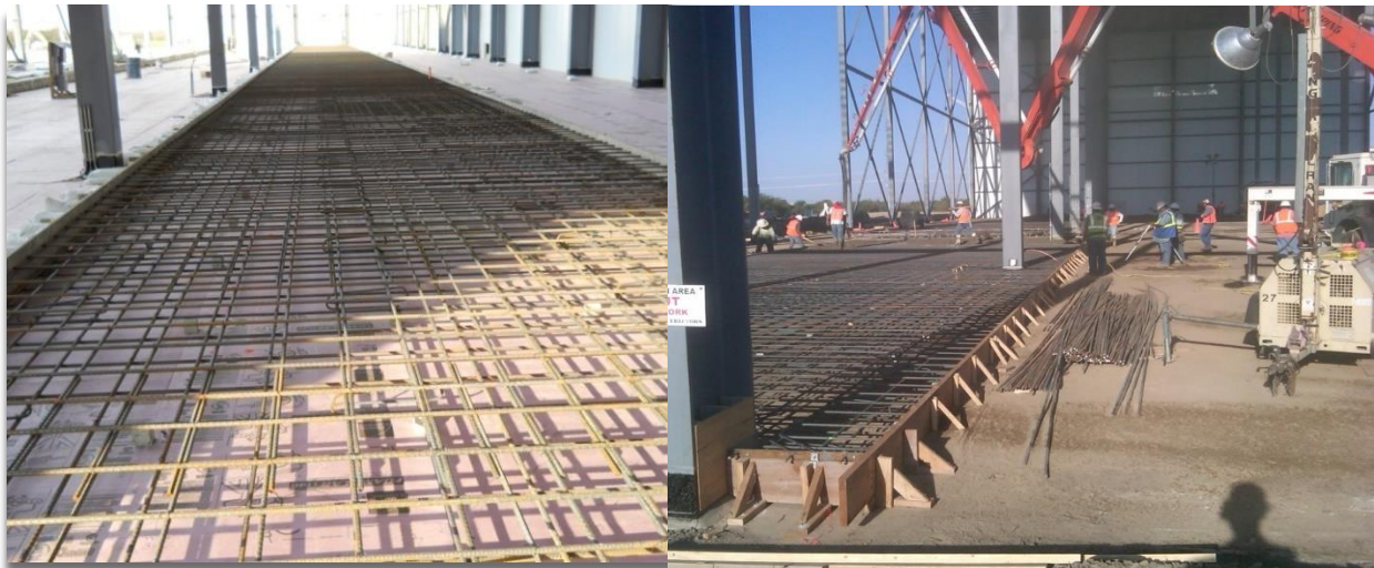
Figs. 45 & 46, Reinforces slabs that support racking that supports roof and braces walls (ACI 318 foundation design required). -15F freezer on left on insulation. 34F refrigerated space on right without insulation.
