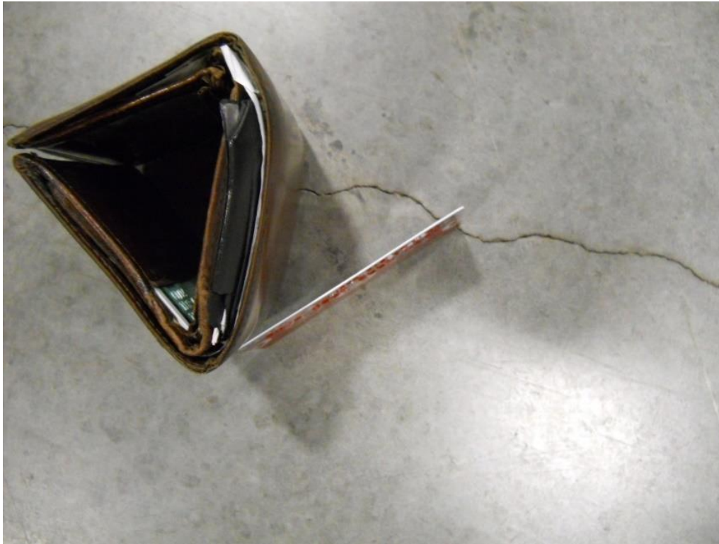
Fig. 19, Typical largest crack in a continuously reinforced high speed travel aisle
