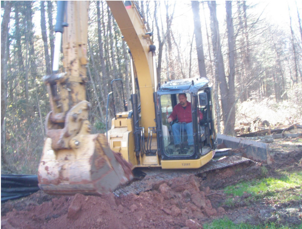
Track Hoe Excavator stays uphill of the silt fence limit of disturbance.
