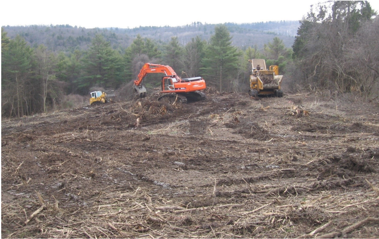
Tree cutting and chipping operation on the author's company's approved housing site.
