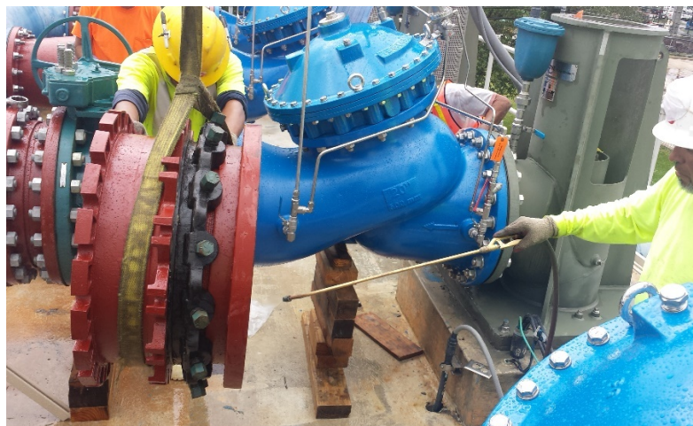
Figure 14: Examples of spray disinfection for pipe components being replaced on an existing finished water pump station. After being sprayed, the wetted surfaces should not be handled, and workers should wear rubber gloves.
