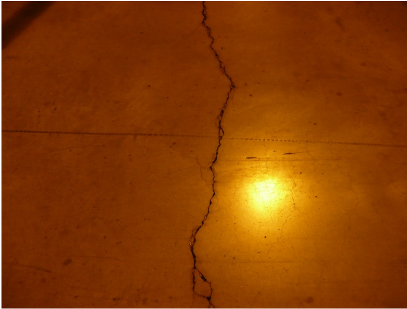
Fig. 18 - Slab crack in a newer facility
