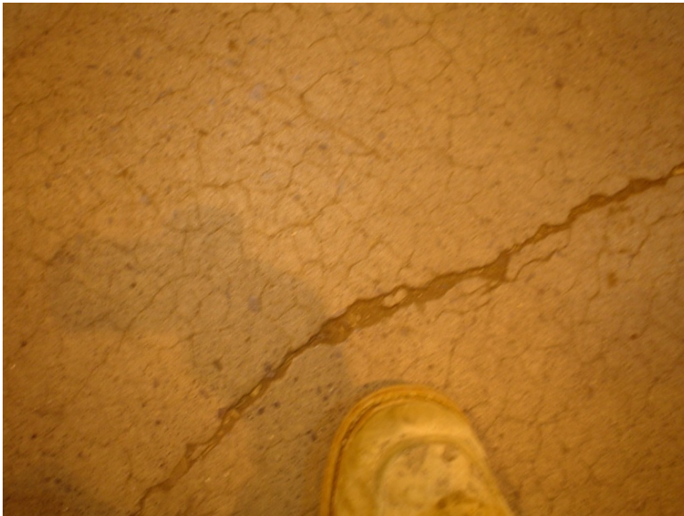
Fig. 19 - Slab crack and joint degradation in an aging facility
