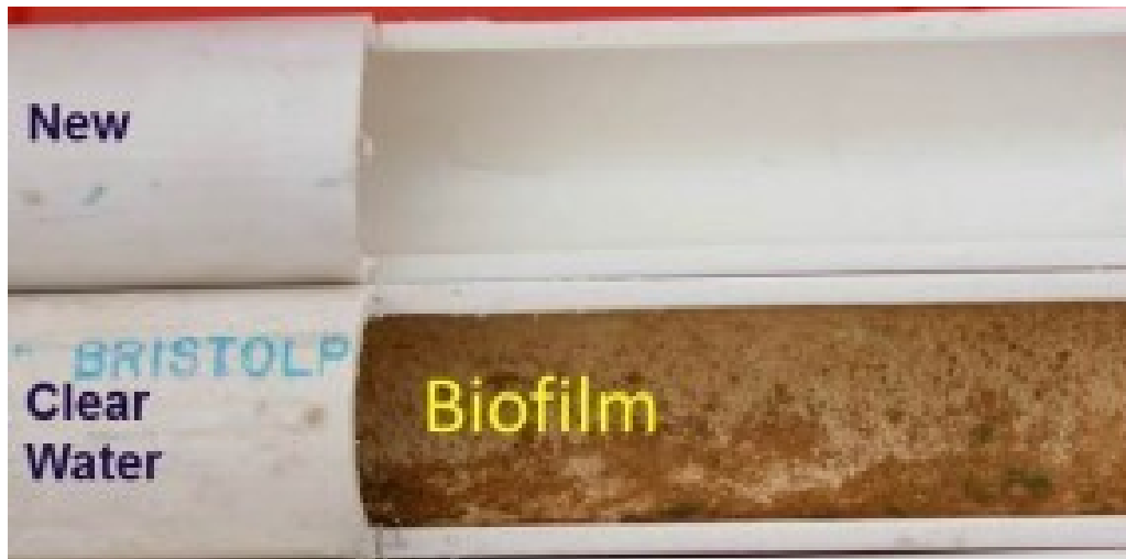
Figure 22: Brand new small PVC pipe (top) and pipe that was in service with brown biofilm growth (bottom).
