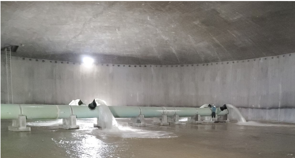
Figure 26: A passive mixing system with several nozzles that are spaced and oriented to mix the entire tank contents.
