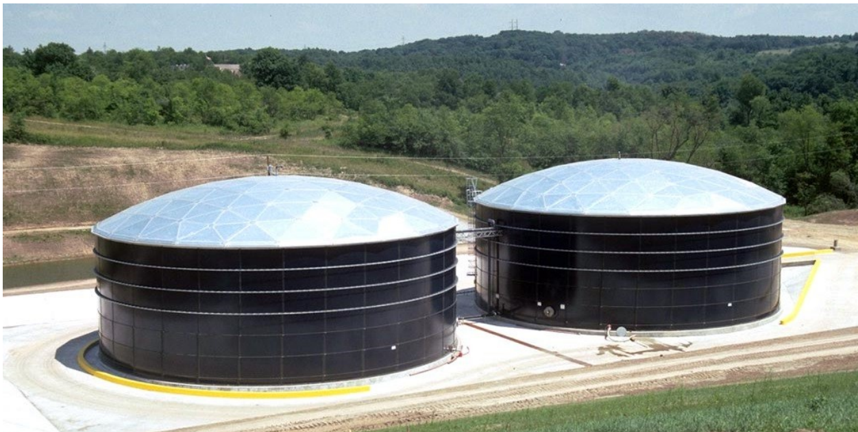
Figure 27: Two ground storage tanks in parallel. Either tank can be taken out of service while the other tank provides the minimum required storage volume.
