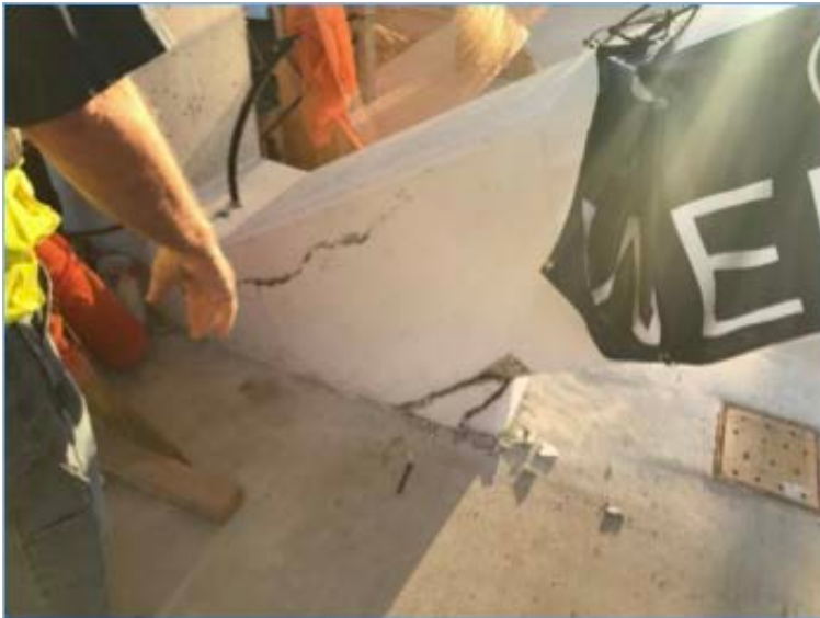
Figure 6 – Cracks at node 11/12 after the main span was set in place over SW 8 th Street and the PT rods in member 11 were de-tensioned.
