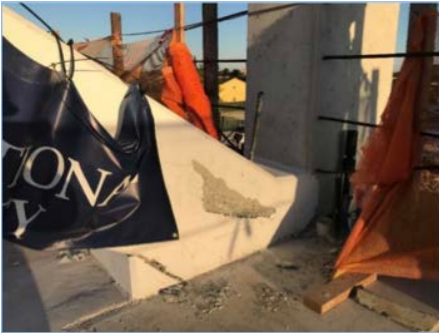
Figure 7 – Cracks at node 11/12 after the main span was set in place over SW 8 th Street and the PT rods in member 11 were de-tensioned.
