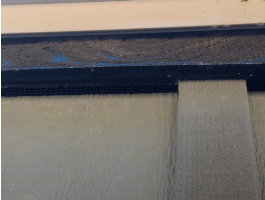
Installed Cor-A-Vent PS-400 strip vent in the overhang of a THOW
