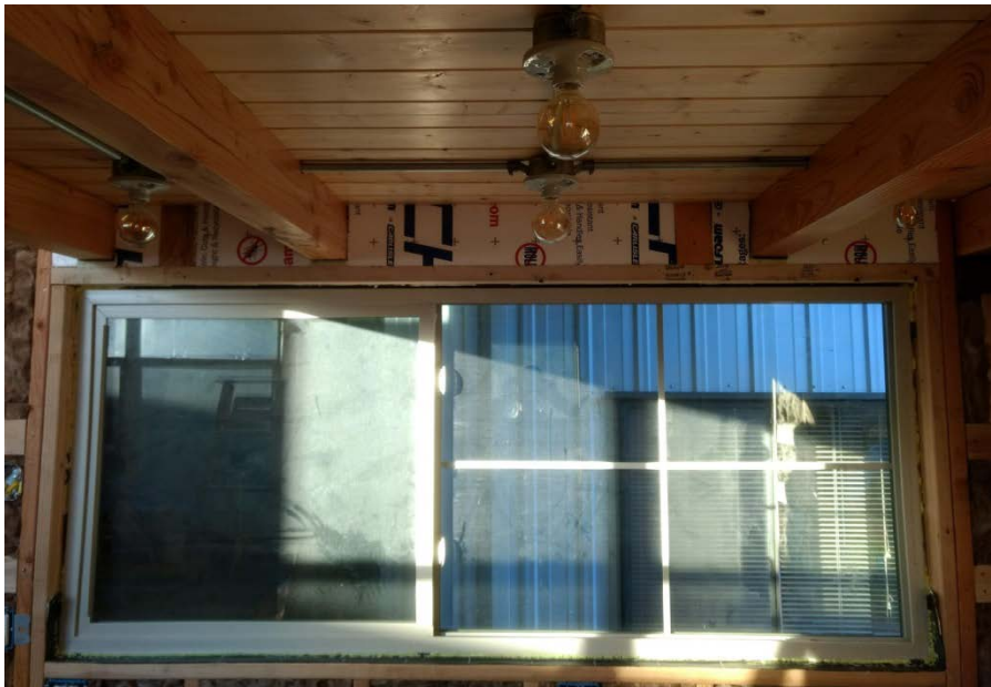
A window utilizing a single member header. This allowed sufficient space for insulating the header with expanded polystyrene rigid foam to reduce thermal bridging.
