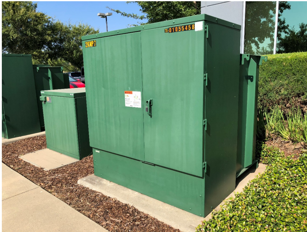
Typical Pad mount transformer
