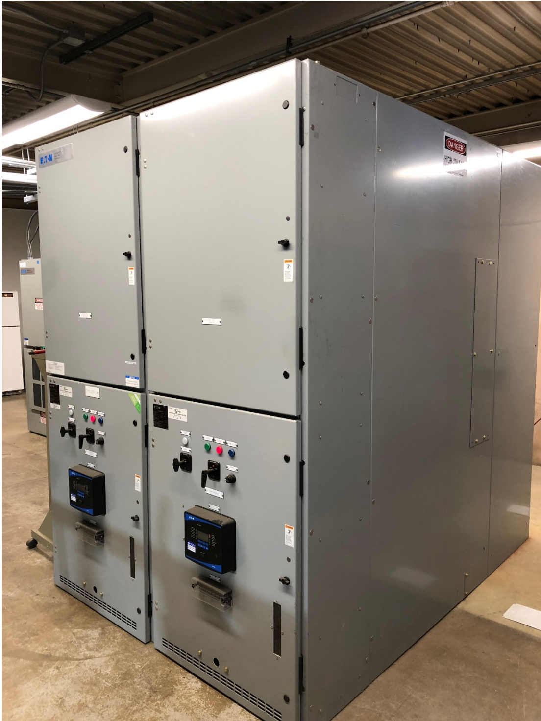
Typical indoor metal-clad switchgear
