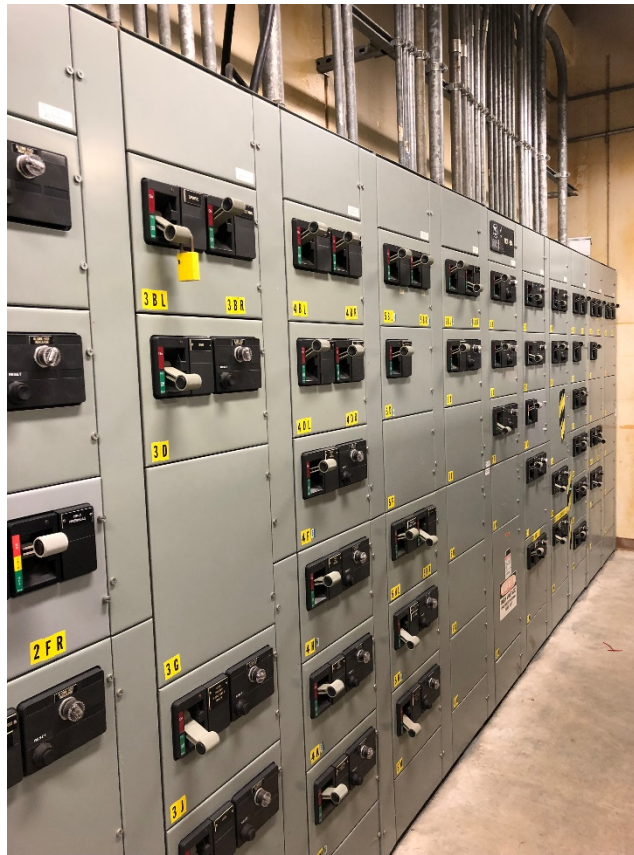
Motor Control Center
