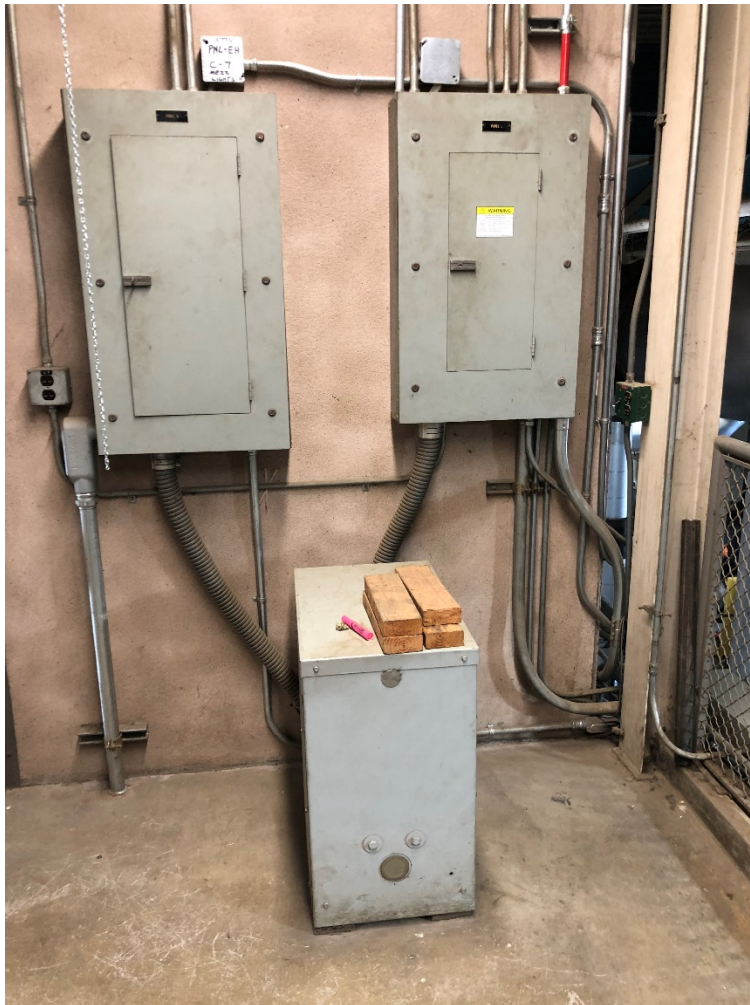
Dry-type transformer feeding panelboards
