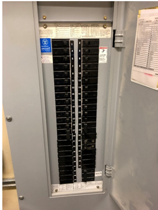
240/120V panelboard and circuit breakers
