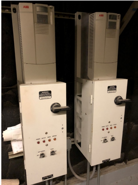
Open air 6-pulse VFDs
