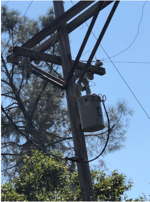
Pole mounted transformer
