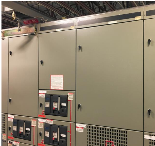
Figure F-3C (A Picture of Switchgear)
