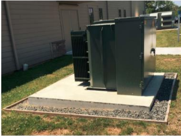
A Picture of a Transformer on a pad
