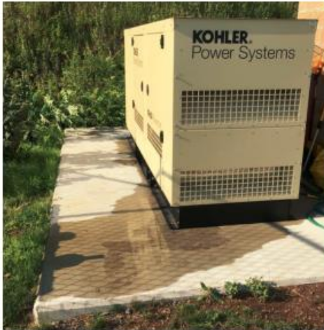
A Picture of an Enclosed Generator on a pad
