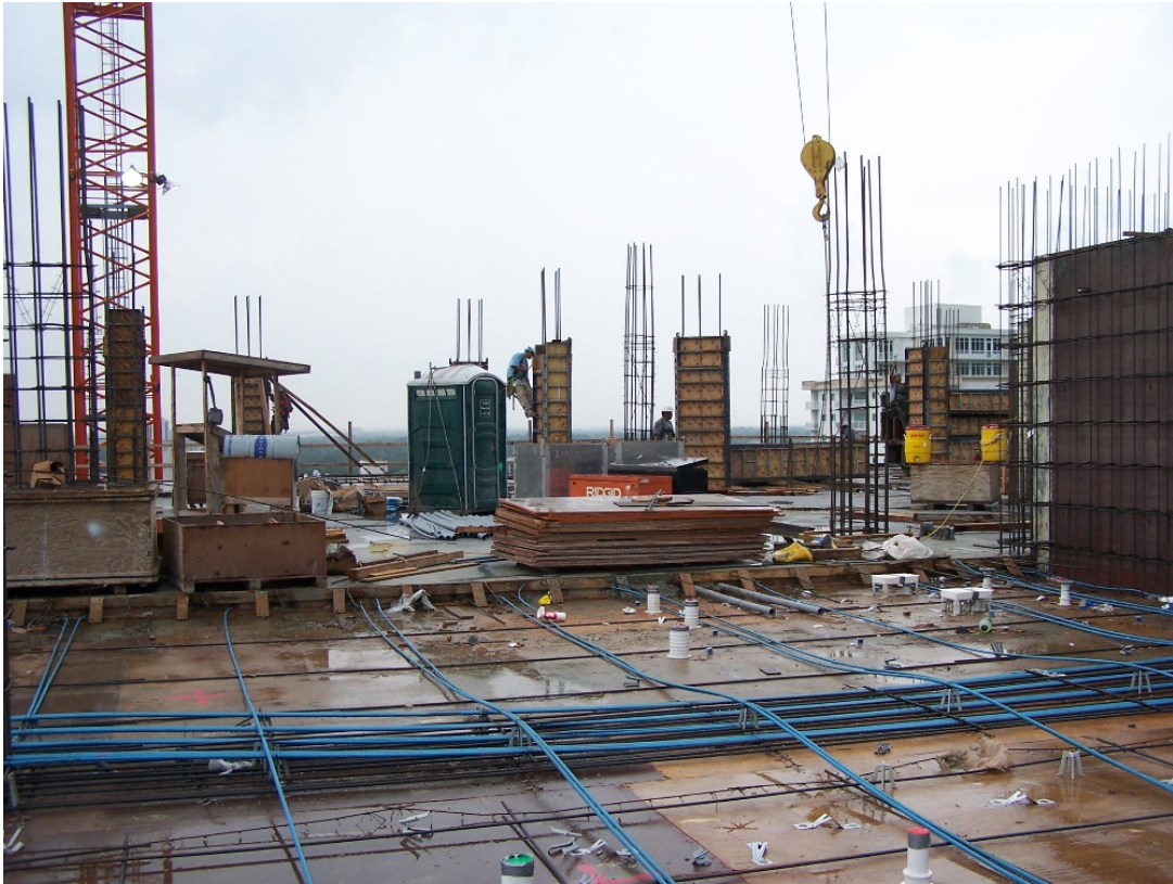
Figure 9. Post-tensioning cables in the slab. Column forms and rebar cages for columns in the background.
