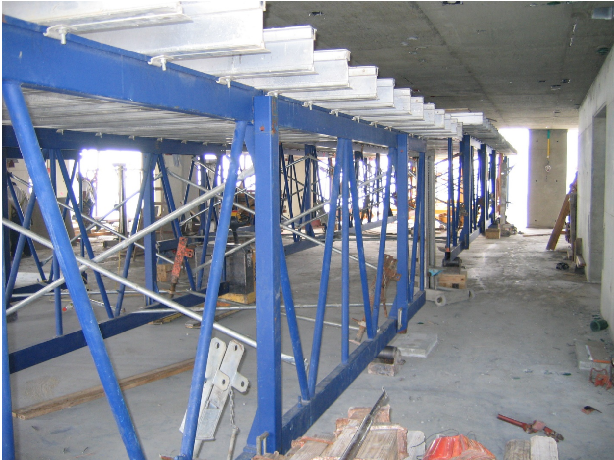
Figure 16: Steel truss tables, with aluminum joists (runners). This table was used as shoring, the floor is now self-supporting, and the truss table has been removed to allow for the floor to be reshored.
