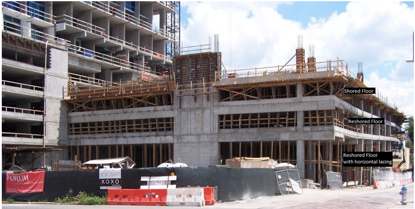
Figure 2: Parking deck under construction with 1 level of shores and 2 levels of reshores extending to slab on grade. Note the horizontal lacing on the bottom level of reshores used to increase the capacity of the reshores.
