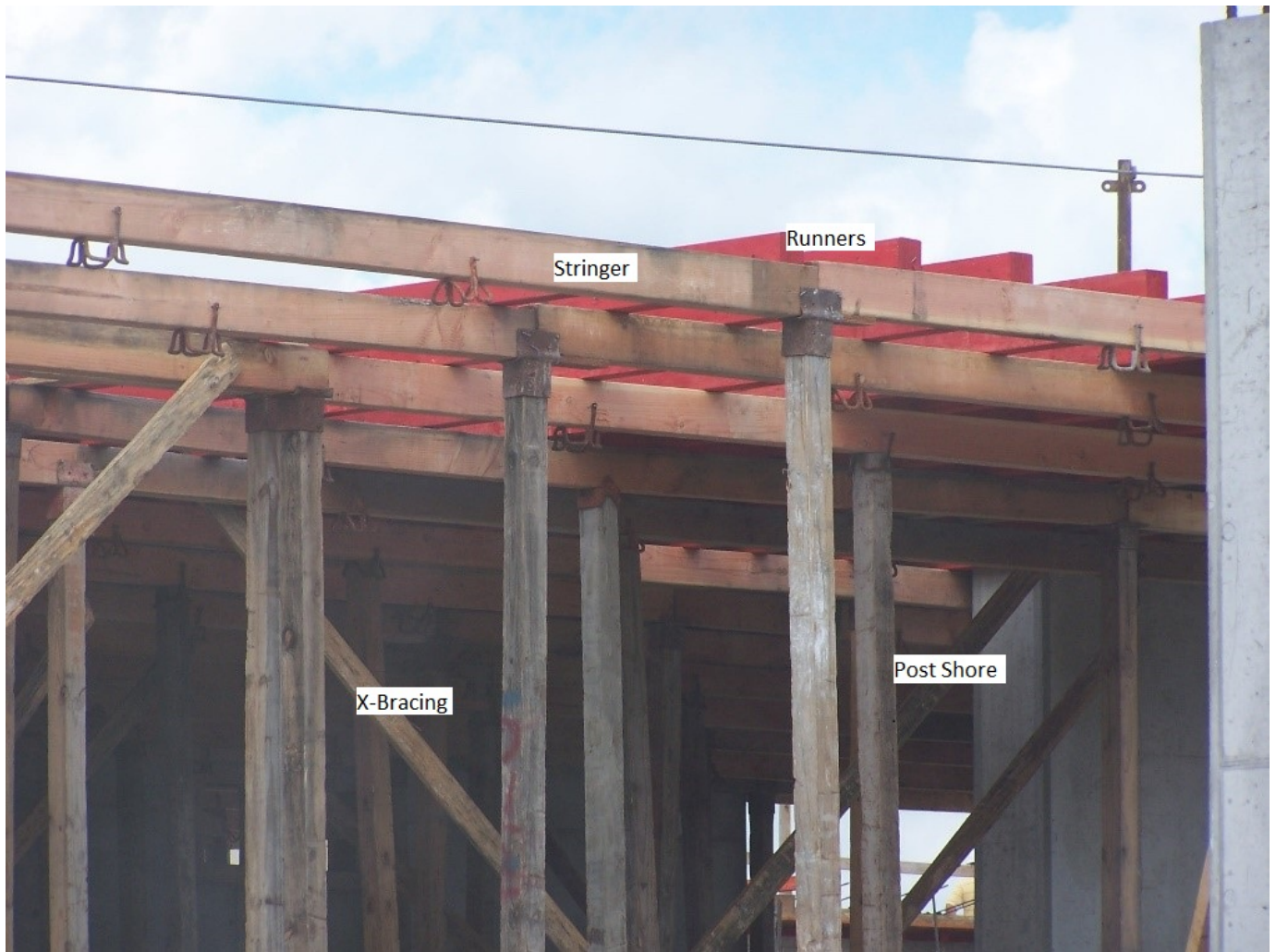
Figure 3. Timber runners, timber stringers, timber shores. Shoring is nearly completed and getting close to being decked with sheathing. B-B Plyform is commonly used as a sheathing material in this type of construction.
