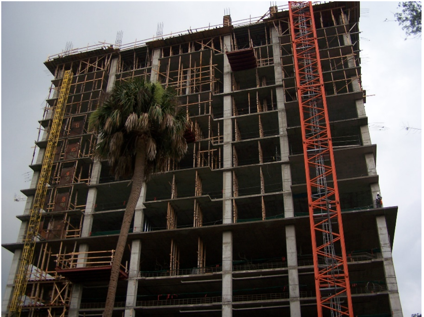
Figure 6. An example of a high rise that required more than 2 levels of reshores due to a non-typical thick slab at the roof.
