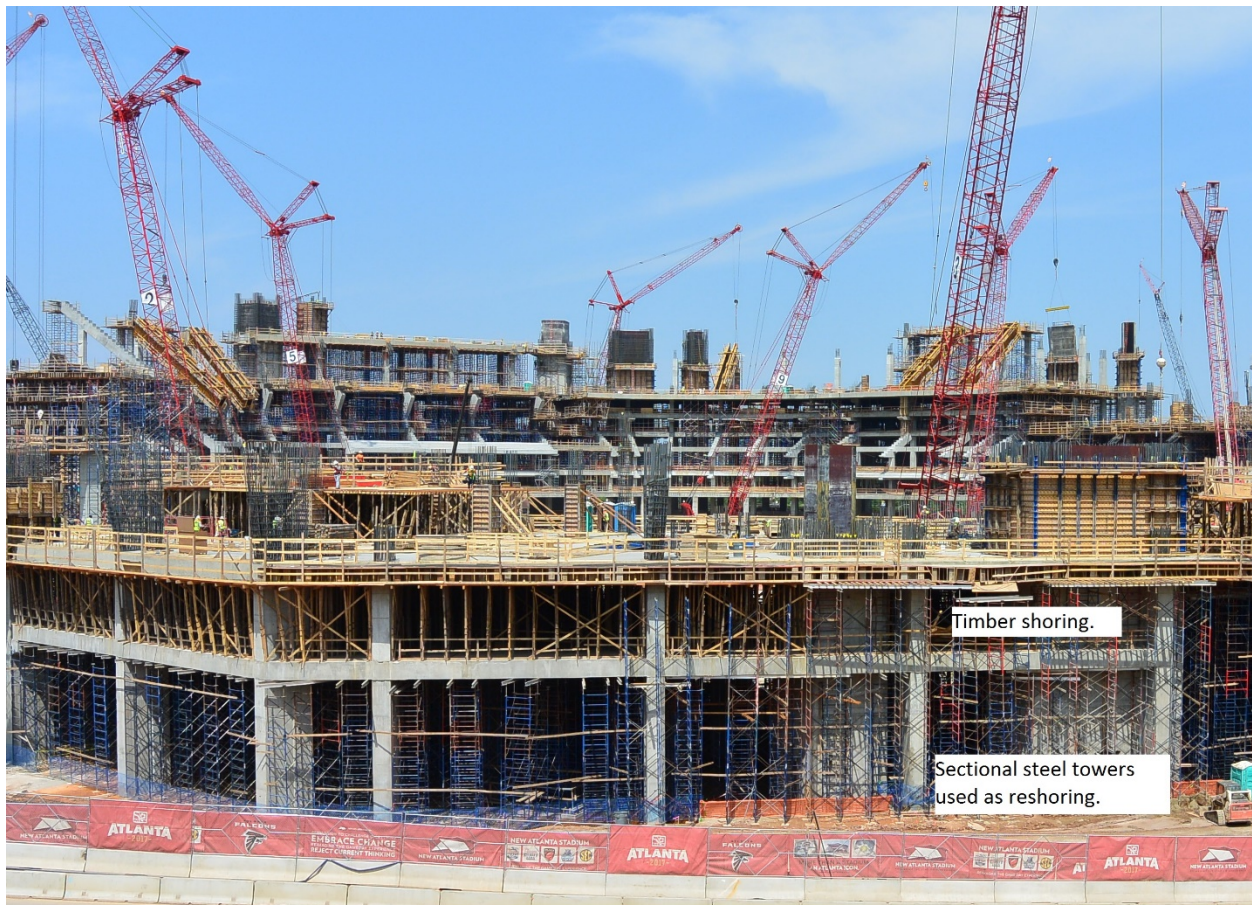
Figure 12. Example of sectional steel shoring towers used for reshoring a tall floor. Timber framing is used for the shored floor. (Photo courtesy of Aluma Systems.)
