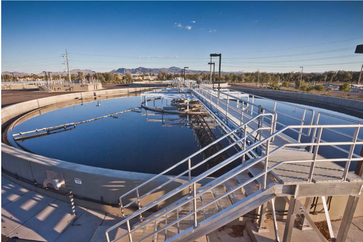
Figure 13 – Clark County Sanitation District BNR Plant Secondary Clarifiers
