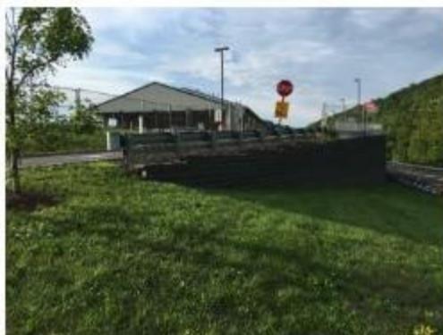
Modular Block Retaining Wall with Steel Guide Rail at the Top
