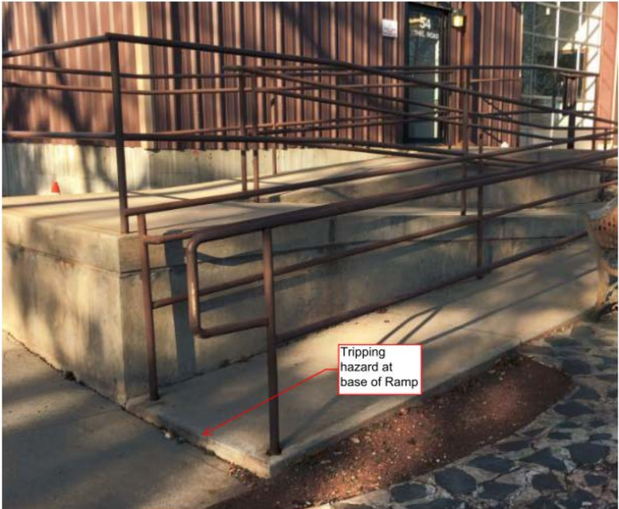
Figure F-12C (Tripping Hazard on an Existing Ramp)
