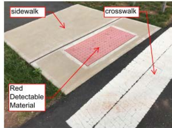
Detectable material at flush end of sidewalk
