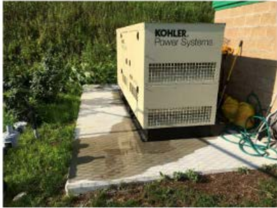
A generator enclosure
