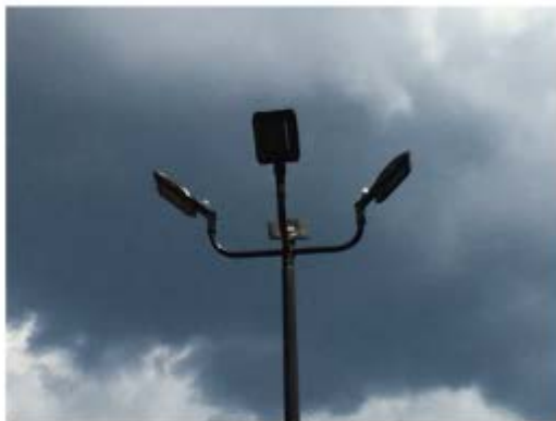
A Quad LED Type Site Light (fixtures set at 45 degrees)
