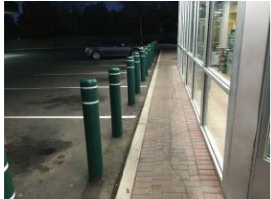
Vinyl covered "decorative" bollards protecting a storefront.
