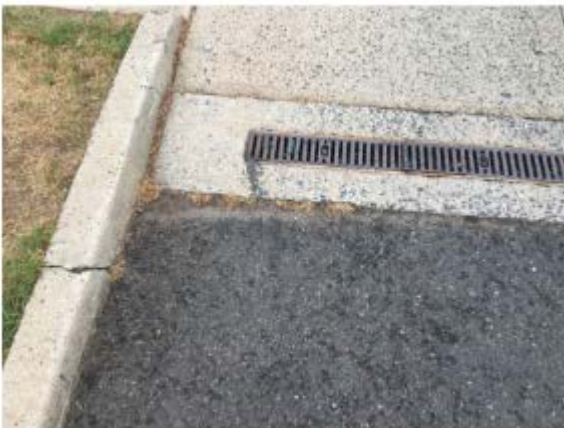
A small 6" trench drain
