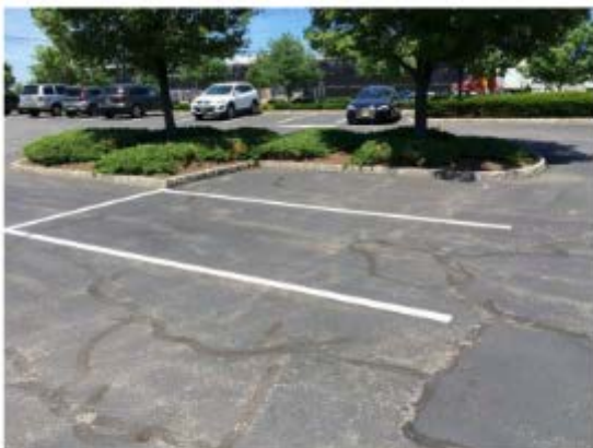
Belgium Block Curbed End Cap for Bay of Parking with Different Length Rows
