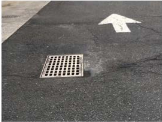
A single cast iron inlet, flush to asphalt
