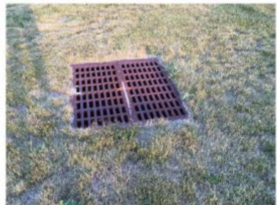
A double cast iron grate inlet in a grassed area
