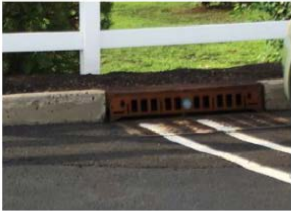
A retrofit water quality plate installed on a standard cast iron curb opening inlet
