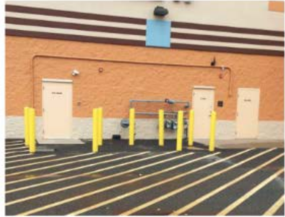
A Gas Utility Manifold with Bollard protection
