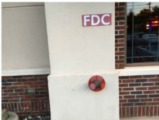
A building mounted "siamese" or dual/twin Fire Department Connection (FDC)
