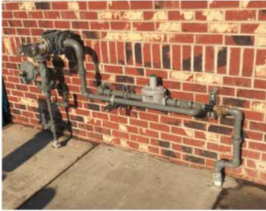
A Gas Utility Manifold
