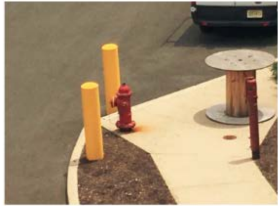
A Fire Hydrant with Bollard protection
