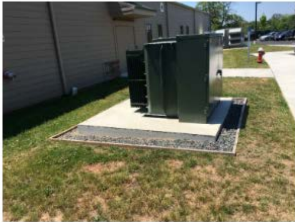
An Electric Utility Transformer on a concrete pad
