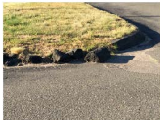
Damaged Asphalt Curb
