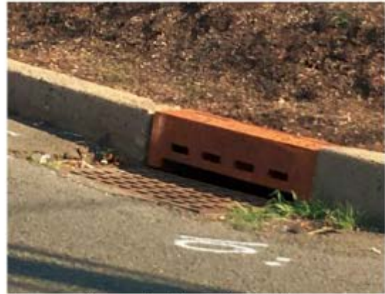
A new standard water quality cast iron curb opening
