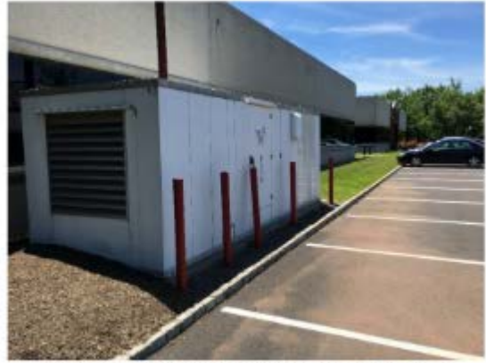
A generator enclosure with Bollard protection
