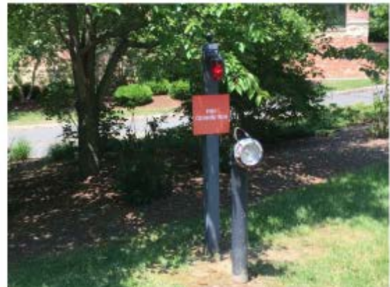
A remote standalone Fire Department Connection (FDC)
