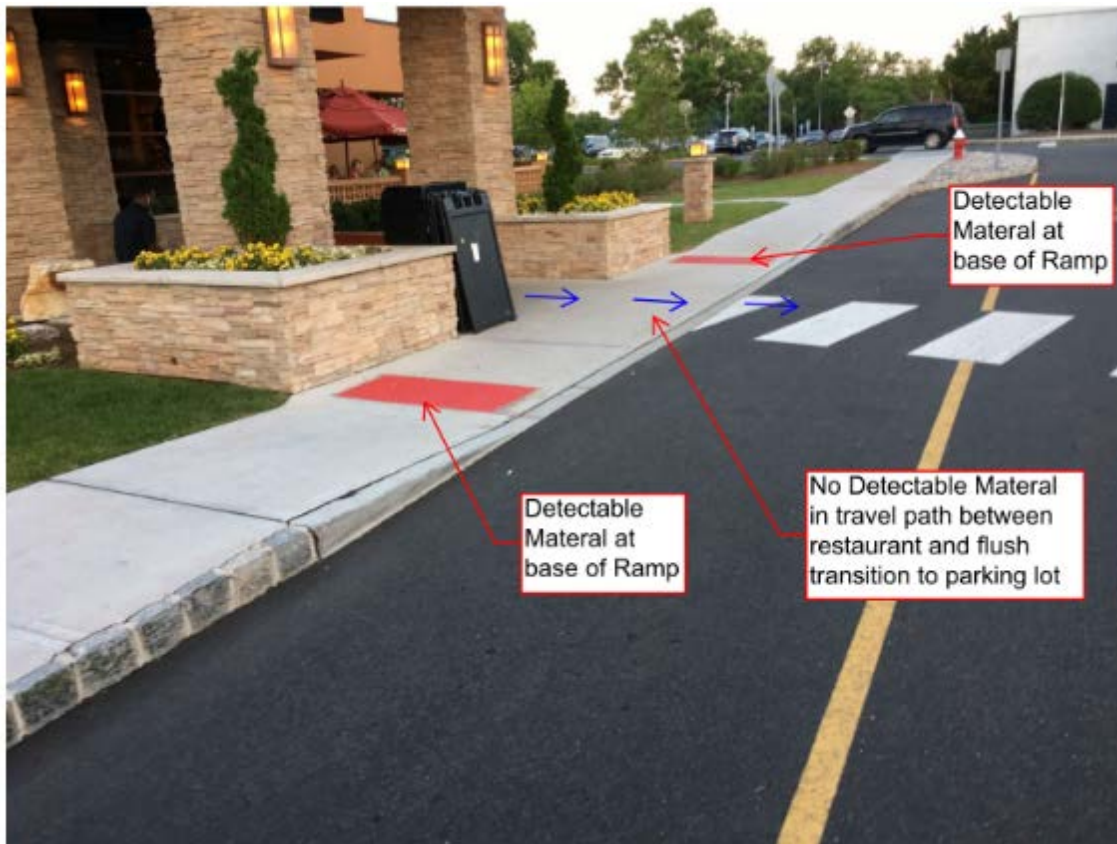
Figure F-13 (Misapplication of Detectable Material)
