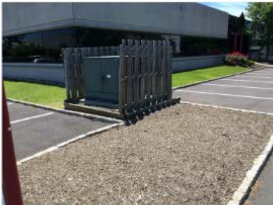
An Electric Utility Transformer with a board on board fence screen
