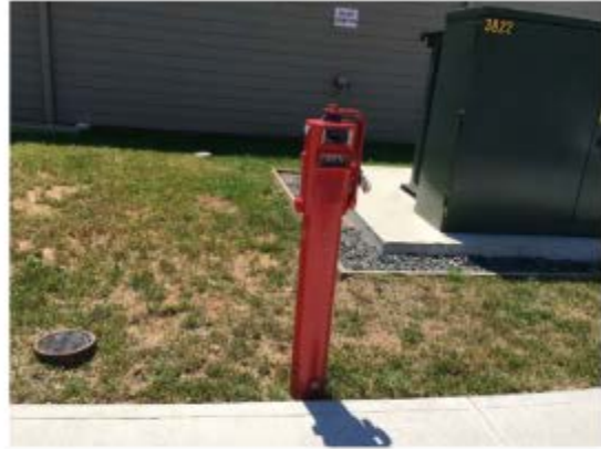
A Post Indicator Valve
