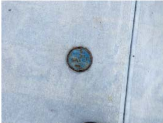
A Water Utility Valve Cap
