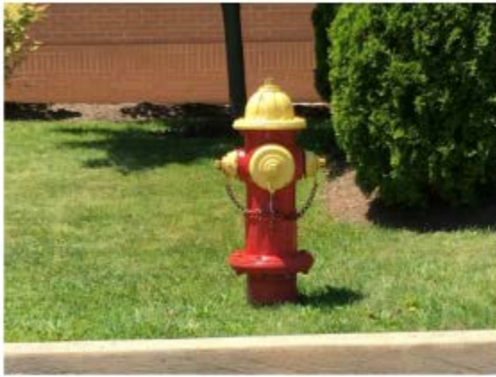
A Fire Hydrant
