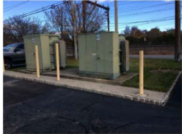
Two Electric Utility Transformers with Bollard protection
