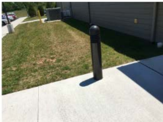
Lighting bollard on sidewalk
