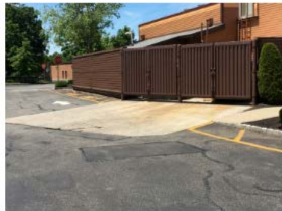
Double Wide Steel Gate Timber Trash Enclosure Integral to Building
