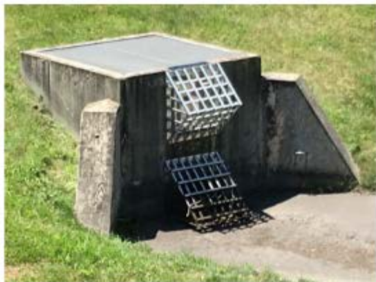
An outlet control structure with cages over the orifices and wing walls on the sides
