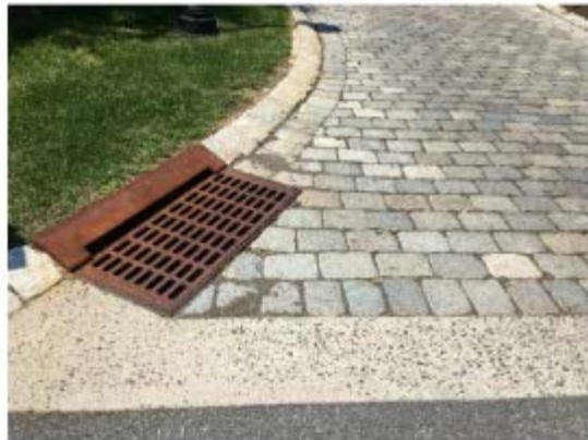
A cast iron grate curb inlet with mountable curb piece
