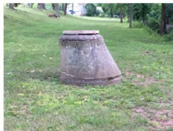
A "concentric" sanitary manhole in a flood plain
