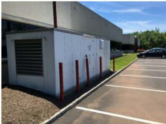
Steel tube bollards protecting an equipment enclosure.
