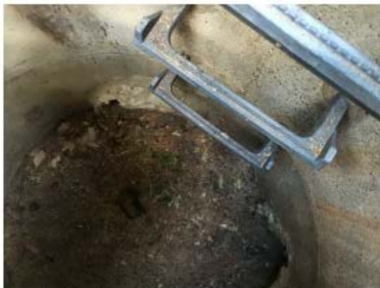
Inside of a manhole showing the ladder rungs and the drainage pipes
