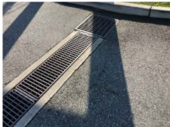
A 12" trench drain with an area drain outfall
