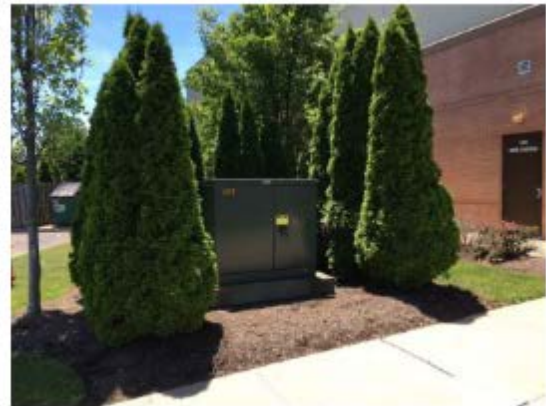
An Electric Utility Transformer with landscaping screening
