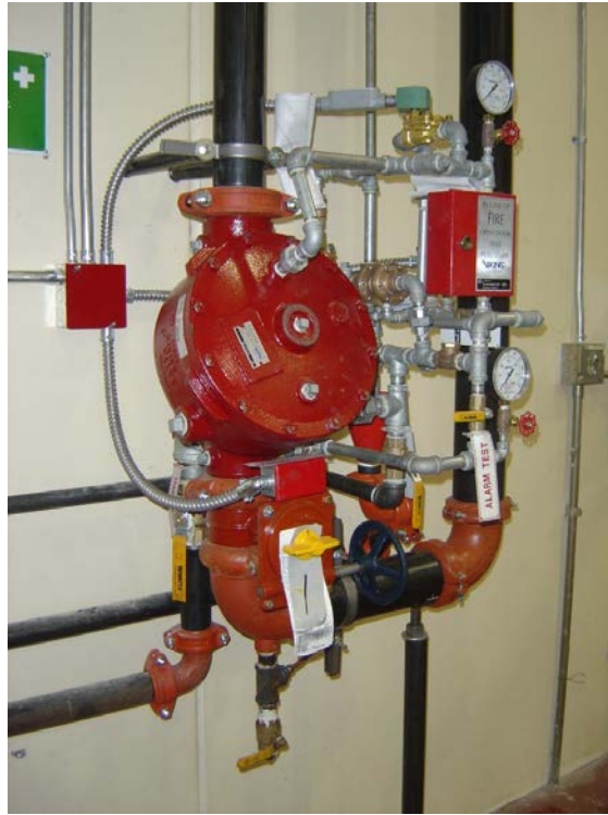
Figure 13 - A Fully Trimmed Alarm Check Valve
