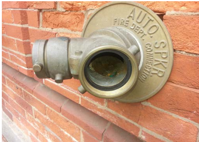
Figure 14 – Typical Fire Department Connection (Note the missing cap)
