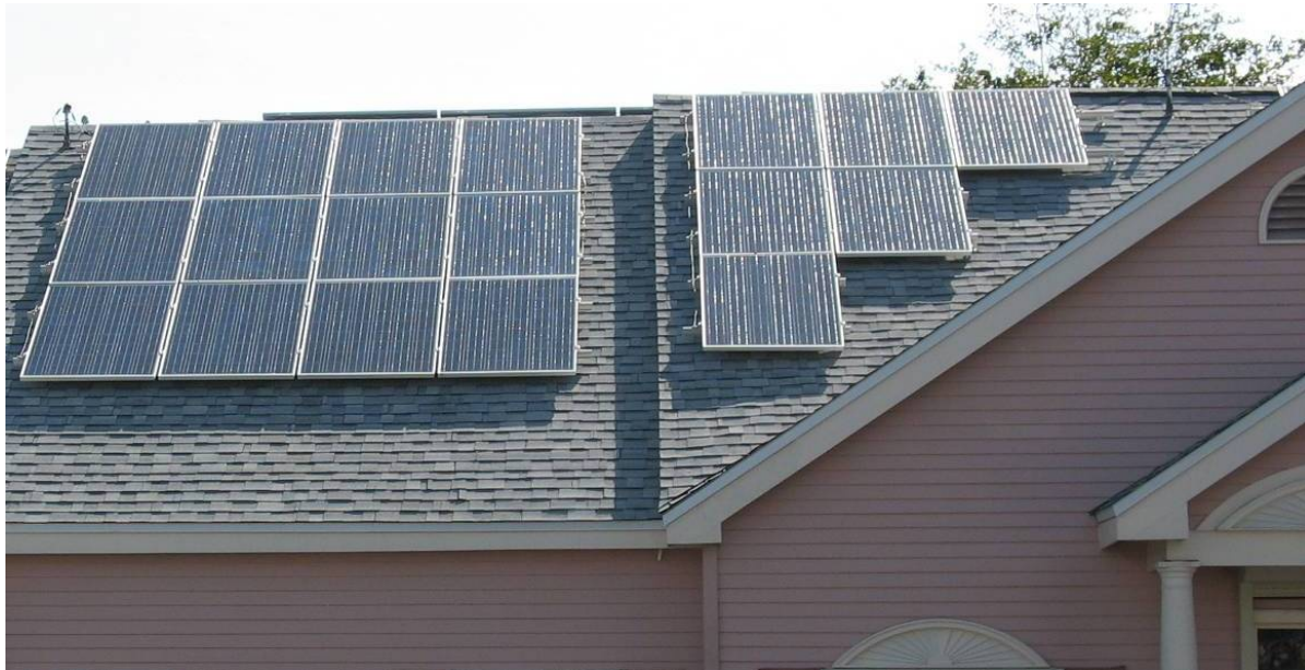
Figure 10 – Roof-mounted solar panels
