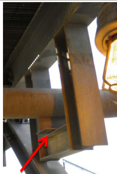
TEE welded to pipe, slides on I-Beam
