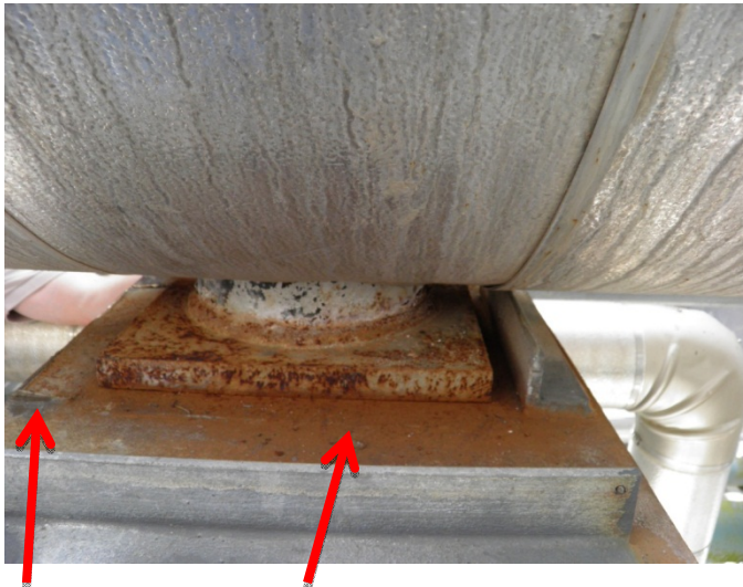
Missing Guide Steel
