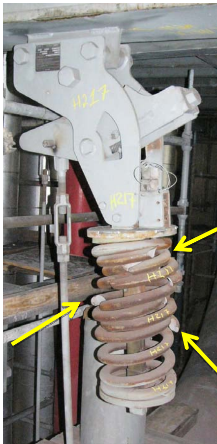
Shattered spring on constant support hanger can. Spring was not passivated properly after acid pickling, and failed due to hydrogen embrittlement.
