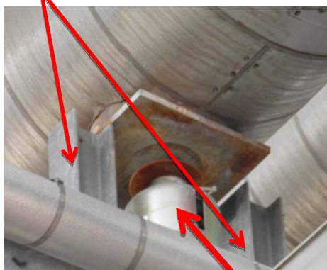
Trunnion w/ plate, resting on guide steel instead of load flange
