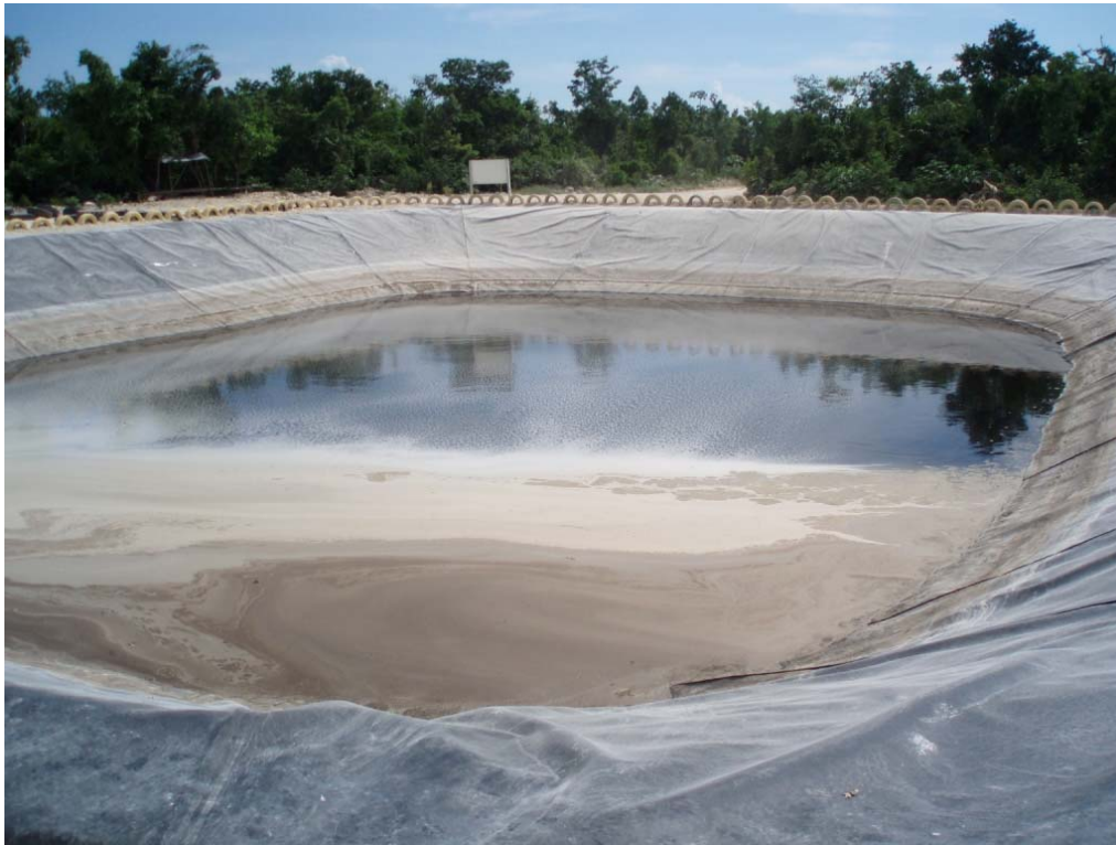
Figure 11 – Geo-membrane Evaporation Pond Liner
