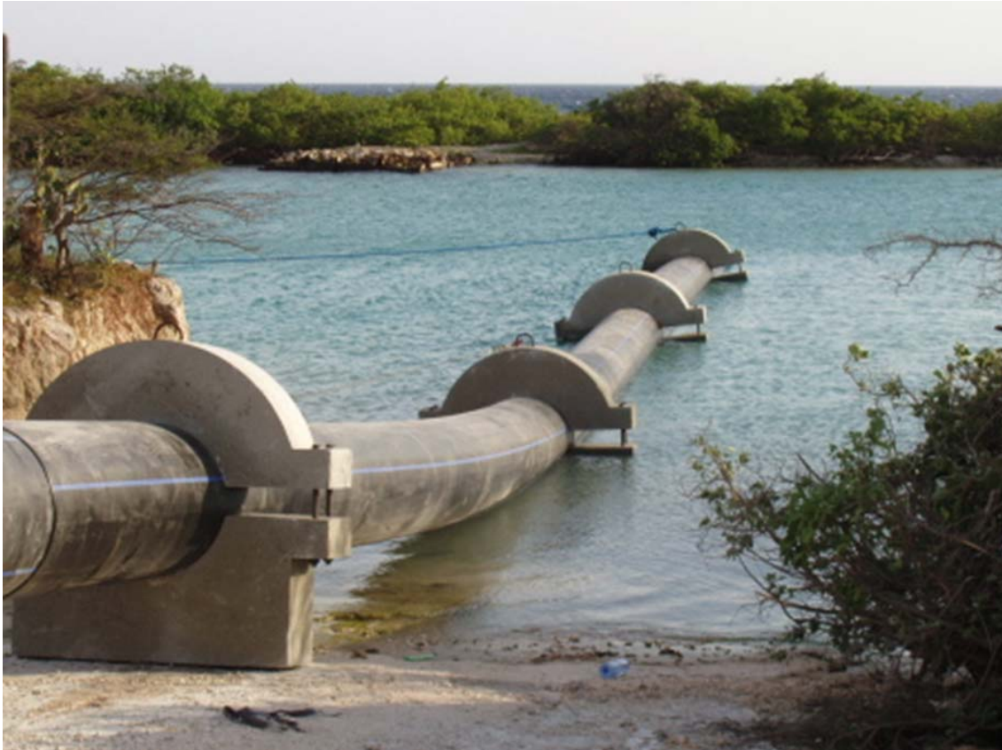
Figure 8 – Concentrate Discharge Pipe
