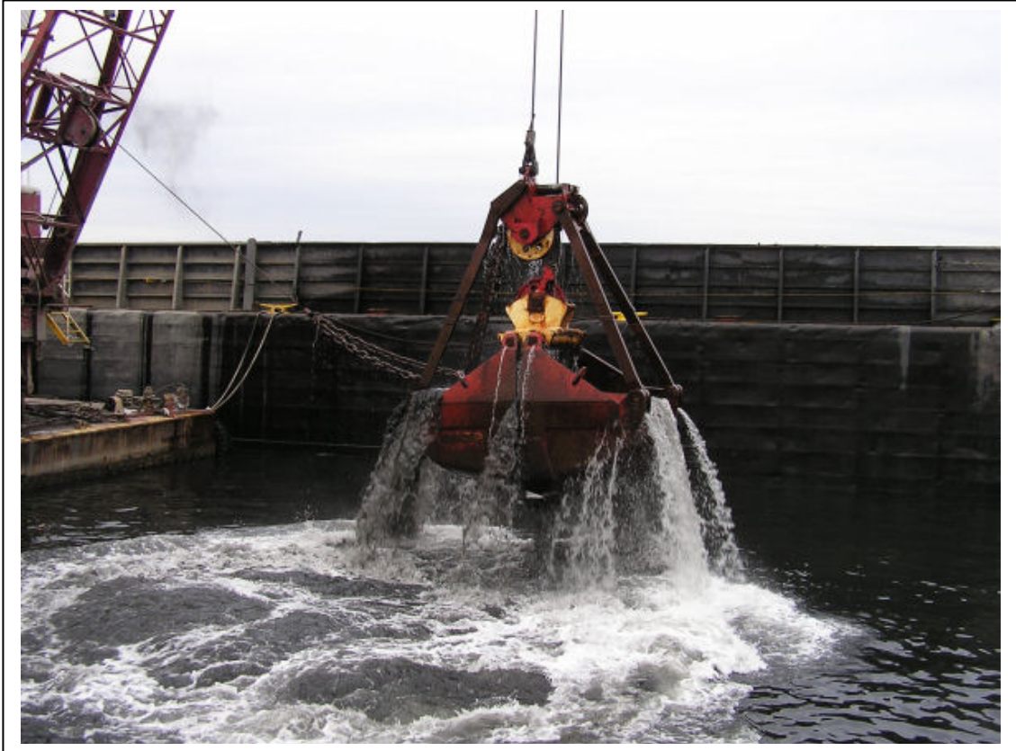
Figure 8b: A Conventional Clamshell “round nosed digging” bucket dredging sandy material – note high volume of spillage
