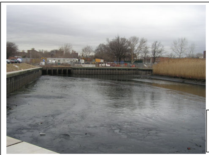
Figure 7a: Common Combined Sewer Outfall "CSO" Outfall, Brooklyn, NY
