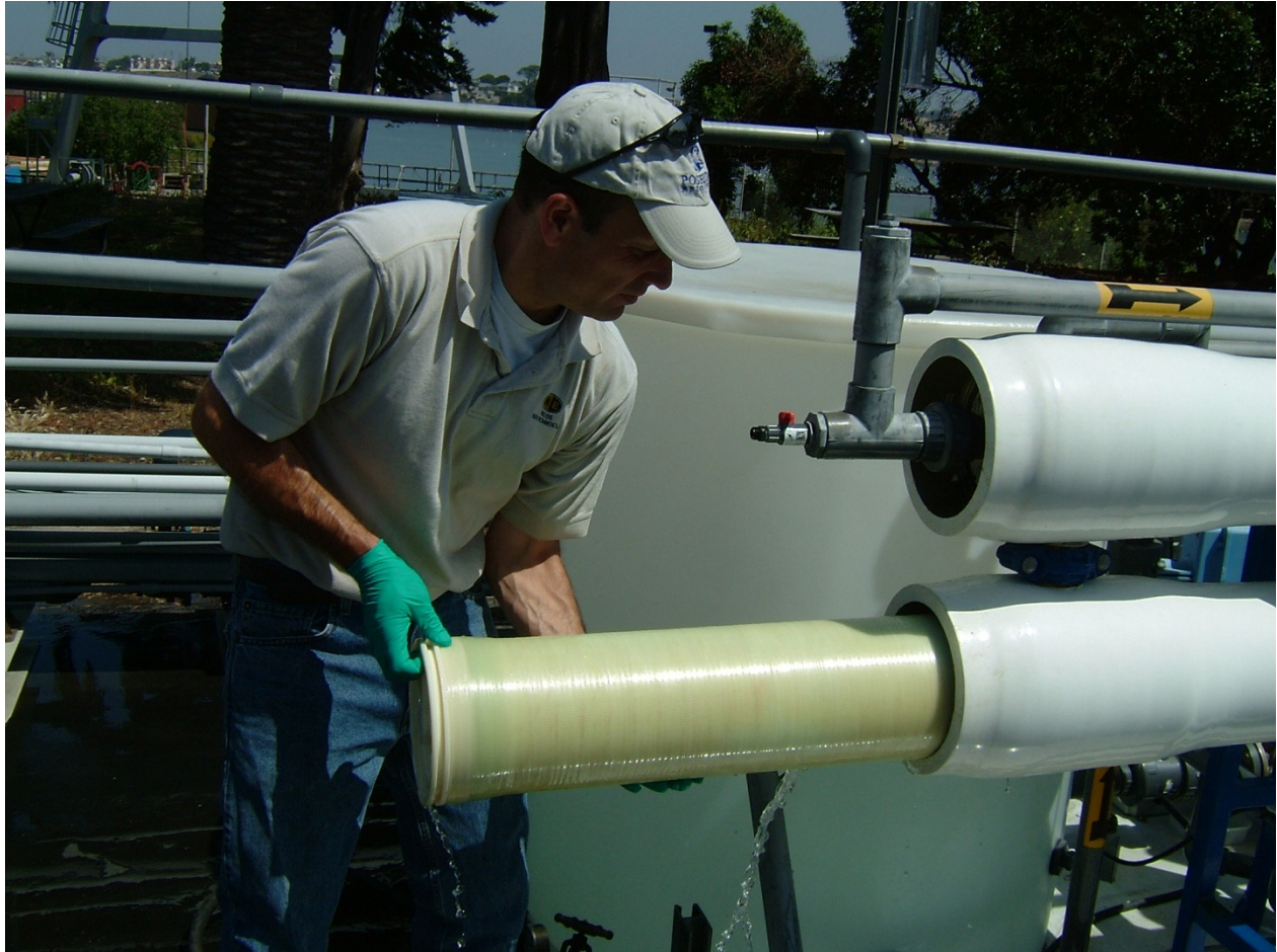
Figure 20 – Unloading of RO Membrane Element from Pressure Vessel
