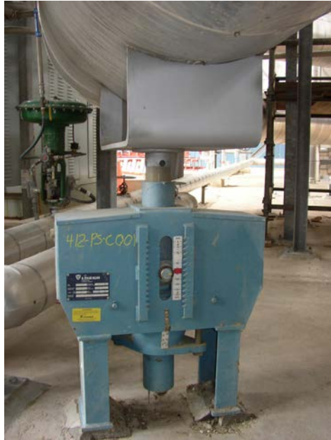
FIGURE 6.7 CONSTANT SUPPORT HANGER FLOOR SUPPORT WITH TOTALLY DIFFERENT INTERNAL MECHANISM THAN OTHERS SHOWN
