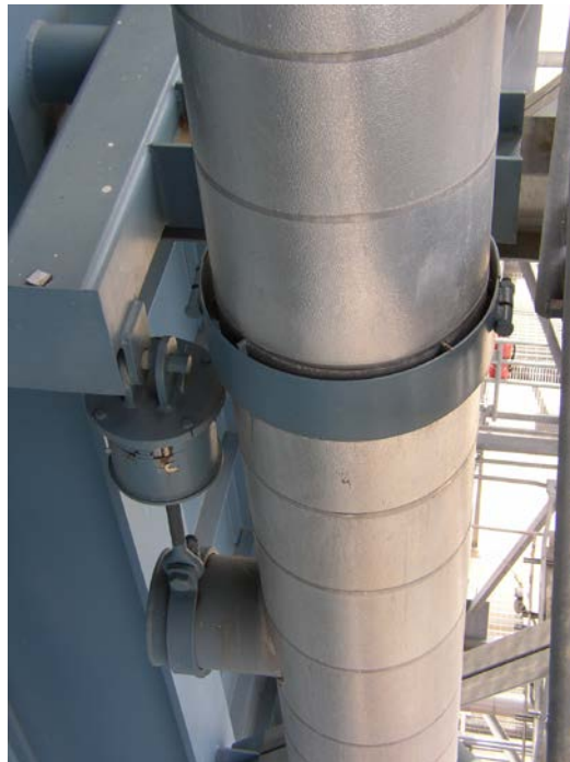
FIGURE 6.10 GUIDE ON RISER PIPE, ALSO NOTE VARIABLE SPRING ROD HANGER ATTACHED TO STACHION BELOW GUIDE
