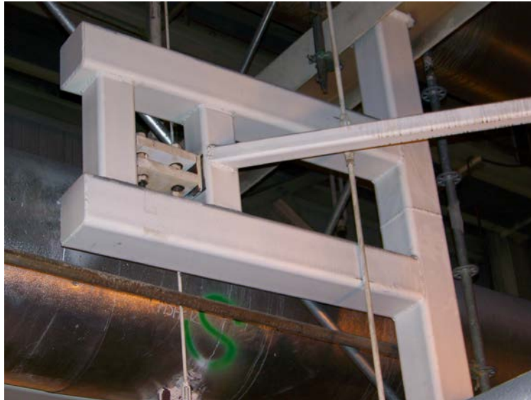
FIGURE 6.11 AXIAL RESTRAINT, (PIPE IS BEHIND STEEL) THESE TYPES OF SUPPORTS TEND TO BE ELABORATE DESIGNS AS SHOWN
