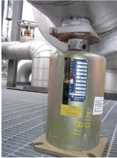
FIGURE 6.3 VARIABLE SPRING FLOOR SUPPORT W/ STANCHION FROM PIPE TO SPRING LOAD FLANGE
