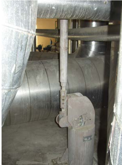
FIGURE 6.6 CONSTANT SUPPORT HANGER, FLOOR TYPE BELOW PIPE; PIPE HORIZONTAL MOVEMENT MUST BE LOW SINCE THIS IS UNSTABLE ARRANGEMENT
