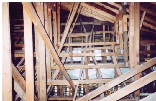
Figure 3: Buckled truss top chord
